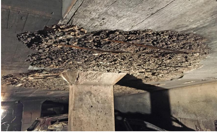
Fig. 1. Explosive spalling damage to a reinforced concrete flat slab in the region of hogging bending moments near a column support following fire exposure in an underground parking structure in Switzerland (2016).
