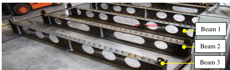
Figure 1. Configurations of cellular steel beams as they are being prepared for the tests
