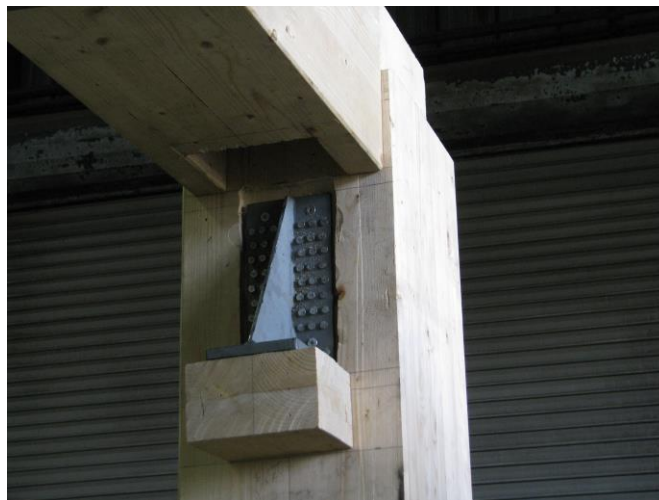
Figure 3 – Project specific connector on column, with routed beam about to be lowered onto the connector. Wooden block at the base provides solid timber seal to the base of the beam. Fire rated sealant yet to be installed.
