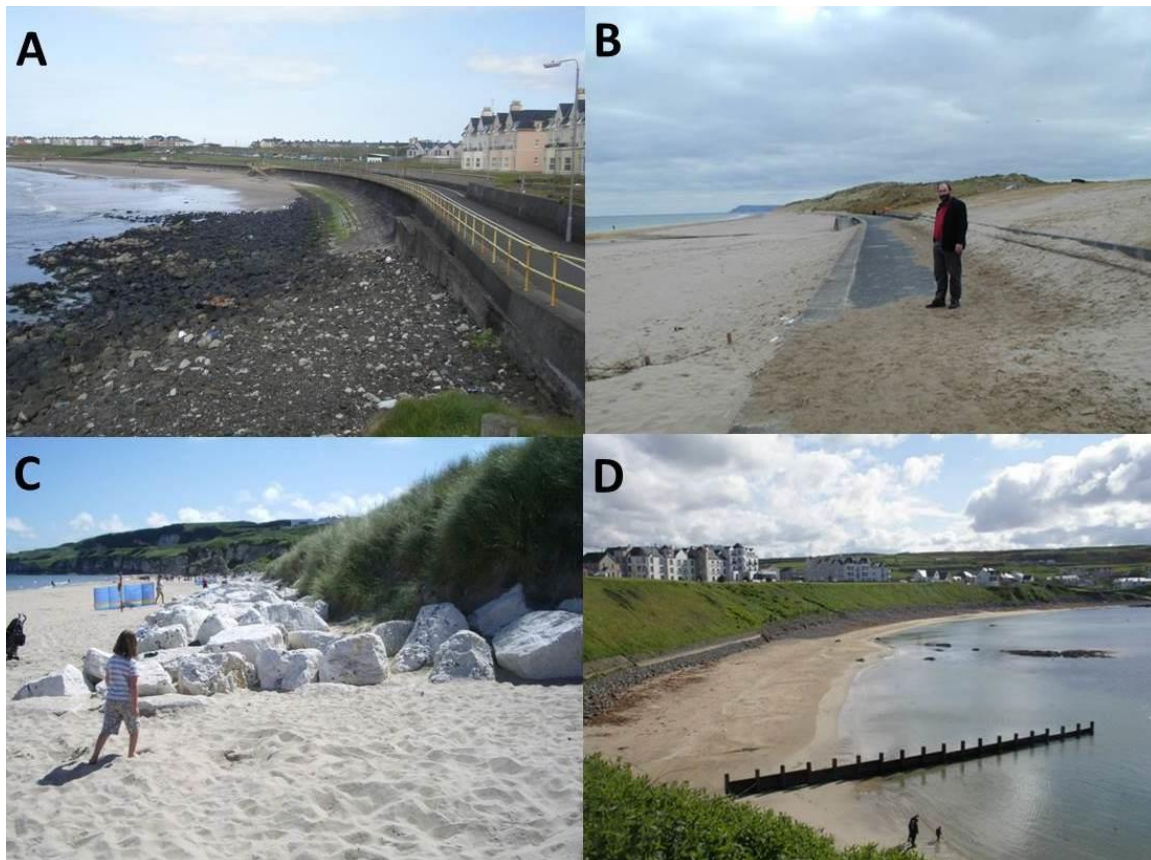
647 648 Figure 3. Sea defences on the north coast. A. Curved seawall and promenade, West 649 Strand, Portrush. B. Seawall and promenade at East Strand, Portrush. This suffers 650 regular inundation with wind-blown sand and requires regular mechanical clearing. C. 651 Rock armour to protect part of gold course. D. Portballintrae groynes ,seawall and 652 stabilized back-beach slope.
