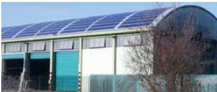
Figure 3. Centrosolar - Thin-film solar plant on the arched roof of a waste sorting station in Monte Crocetta, near Vicenza (40 kWp), constructed in collaboration with Rewatt, Vicenza.
