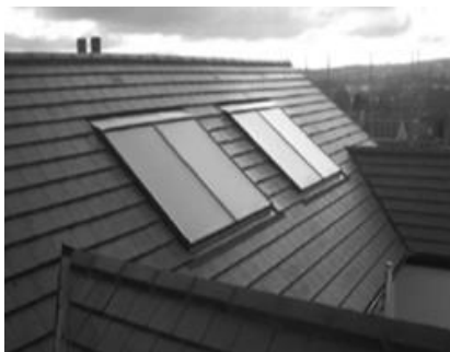
(a) Roof integrated flat plate collectors
