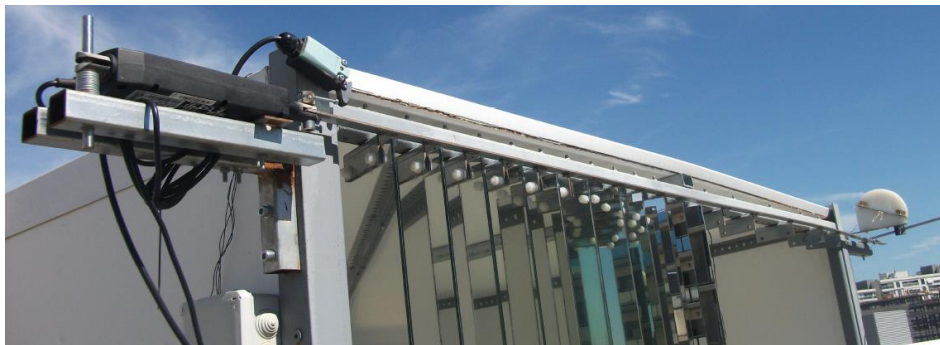
Figure 4. Detail of the implemented tracking system.
