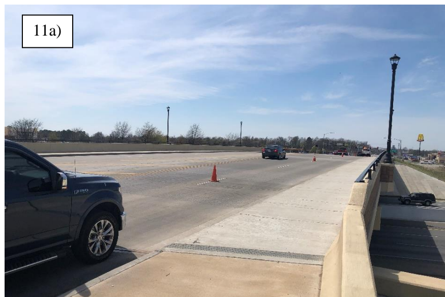
Figure 12. (a) Bridge BB0413 (photo by author) site and (b) map cracking.
