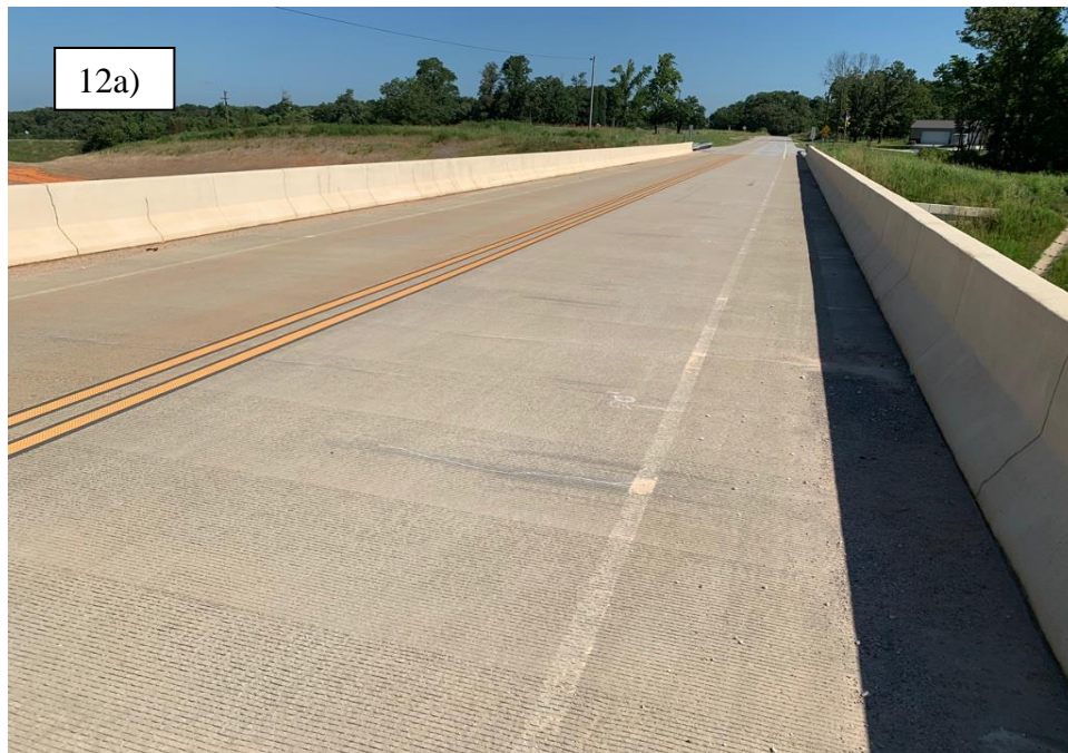
Figure 14. (a) Bridge 07273 site, (b) in-situ crack shapes and (c) map cracking.
