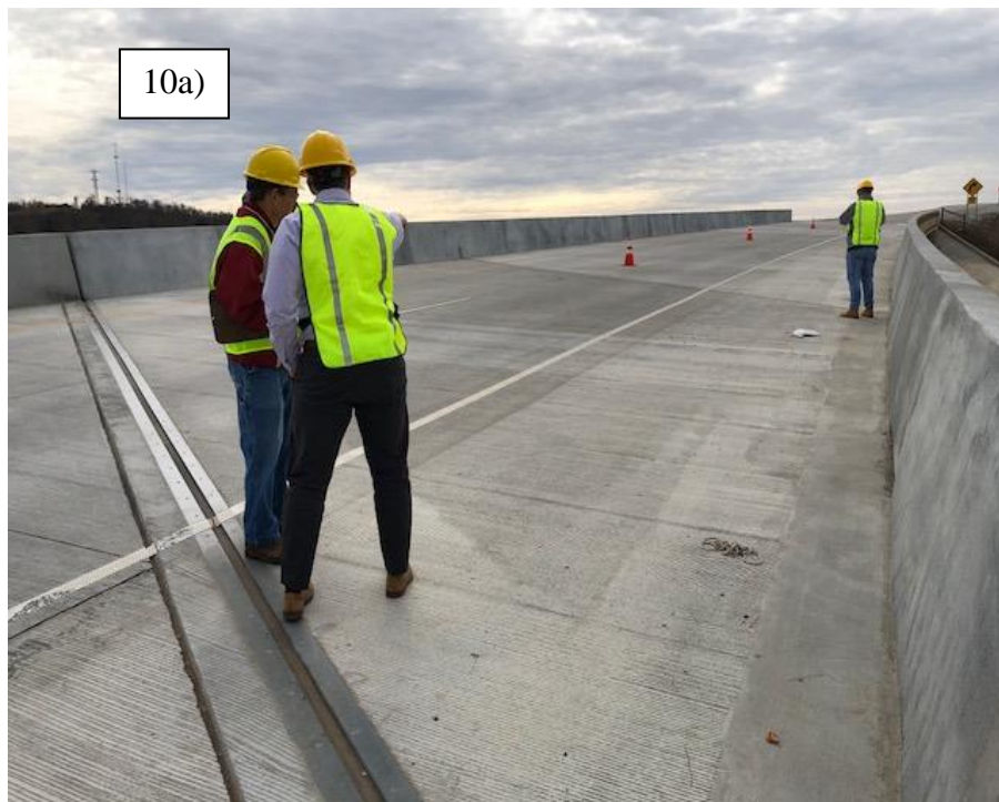
Figure 10. (a) Bridge 07315 site (photo by author) and (b) map cracking.
