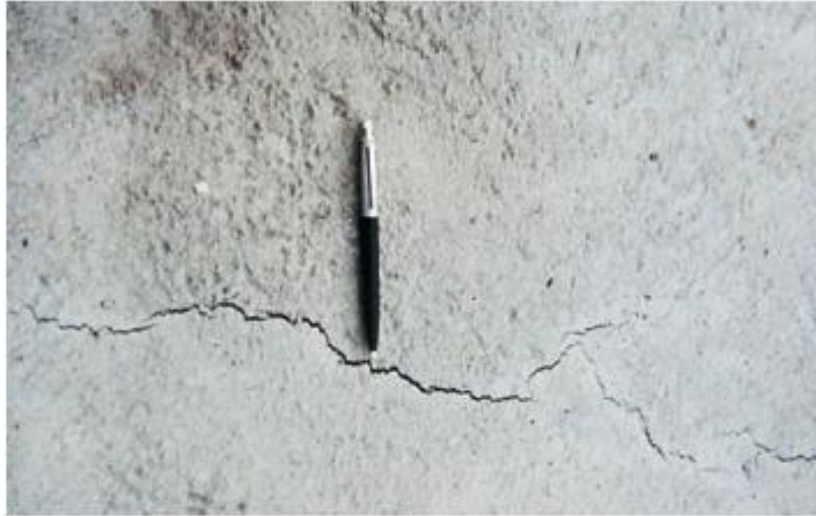
Figure 1. Plastic shrinkage in concrete [15].
