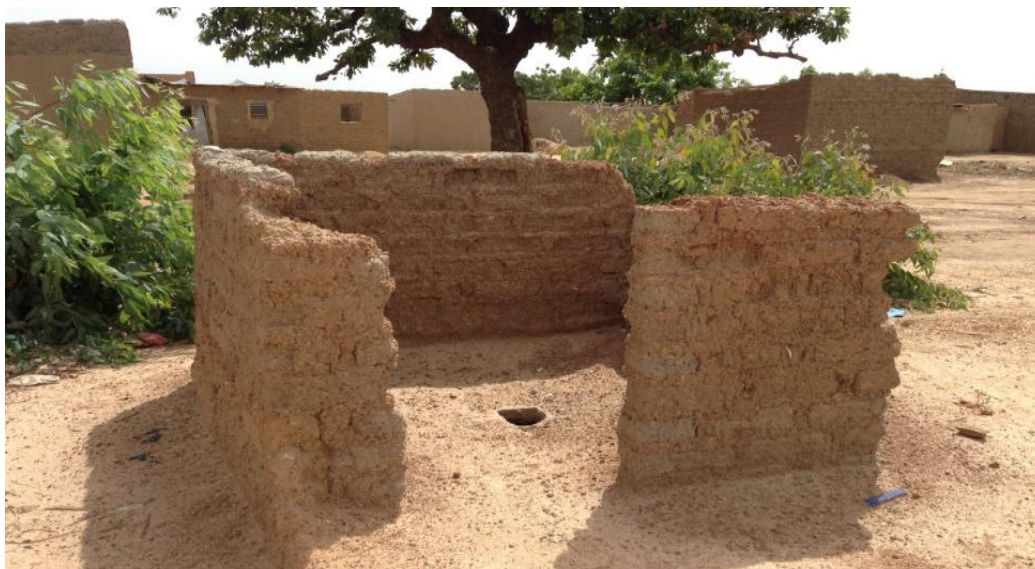
Figure 1. Evidence from Burkina Faso: Toilet before training.
