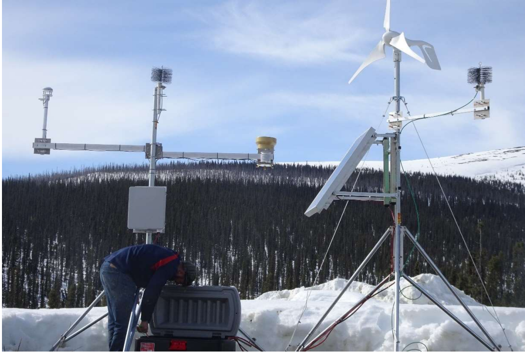
Figure 7 Montana Creek installation
