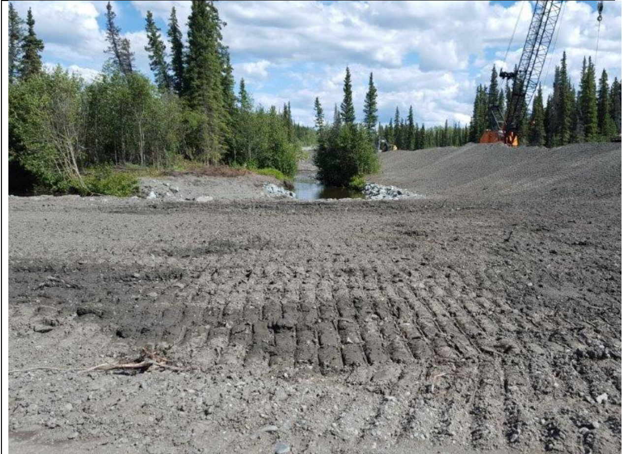
Figure 1.17 Bridge replacement project near Gakona, Alaska. Riprap around stream. Track walking (surface roughening) prior to seed and mulch application.
