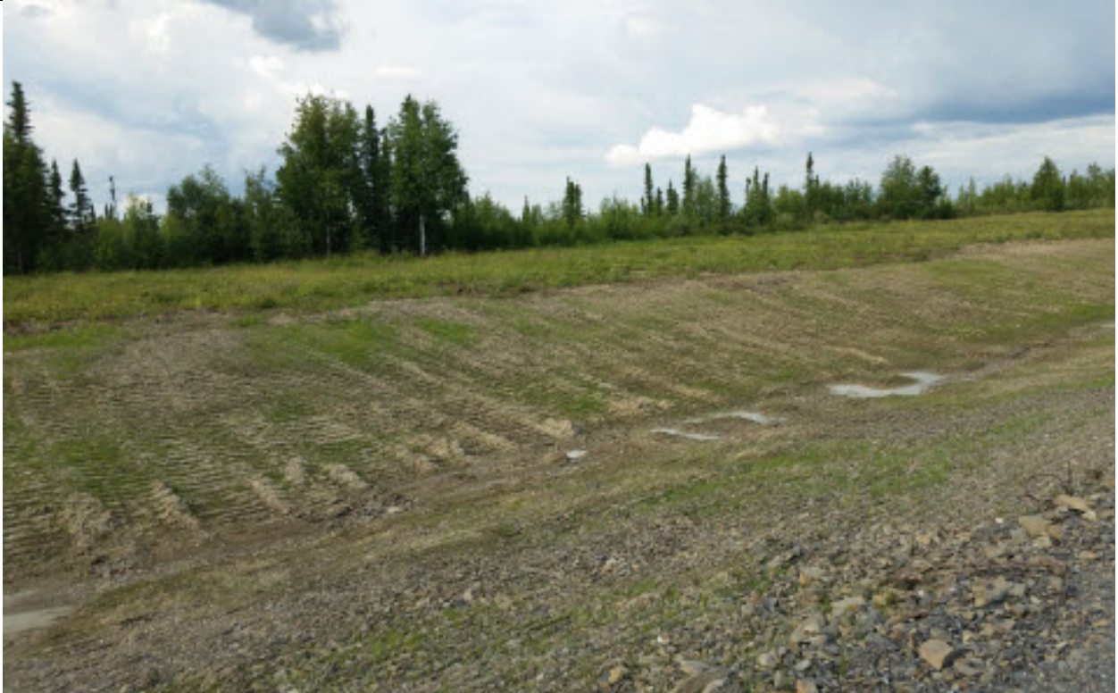
Figure 1.7b Some erosion, sediment in ditch.
