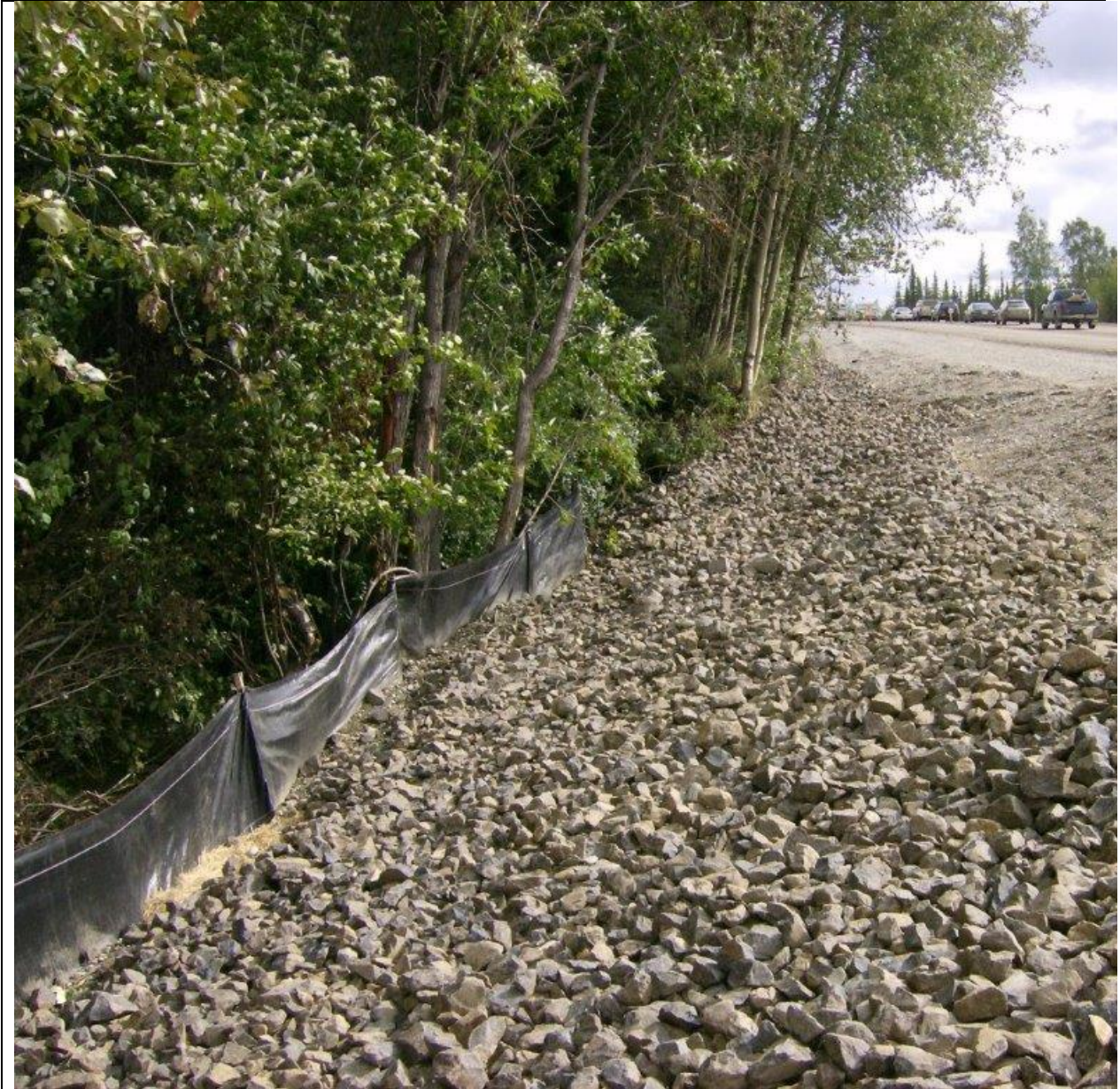
Figure 1.19 Construction project near Fairbanks showing final stabilization (riprap/stone mulch) and temporary perimeter sediment control (silt fence) and surface roughening (grooving) on embankment above placed rock.
