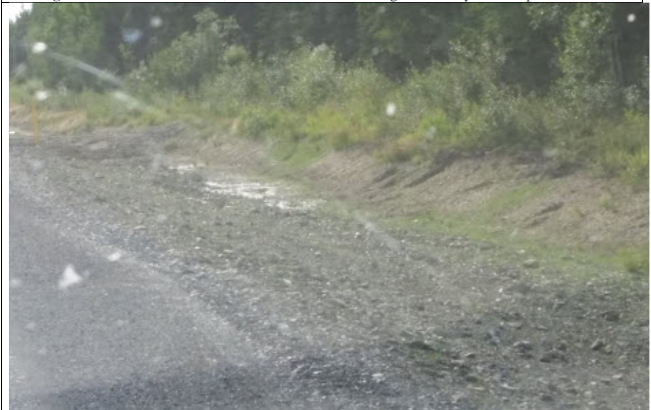
Figure 1.13 Elliott Hwy., recent project. Note erosion on slope and general lack of revegetation. This project has ditch dams (checks) at intervals to inhibit transfer of fines downstream.
