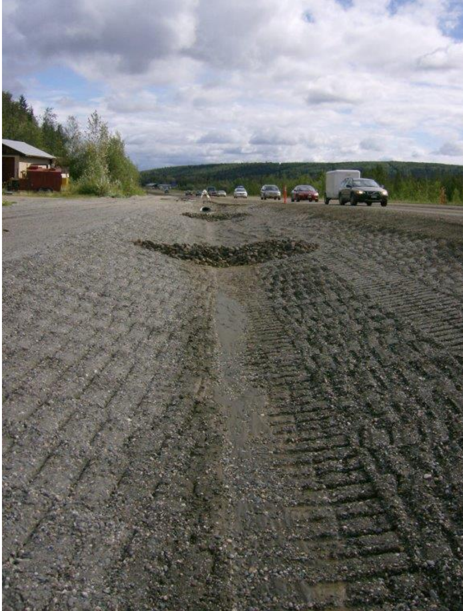
Figure 1.18 Road construction project near Fairbanks, Alaska. Temporary erosion and sediment controls in a conveyance, with surface roughening (grooving on embankments, track walking in ditch bottom) with velocity dissipation (rock check dams).
