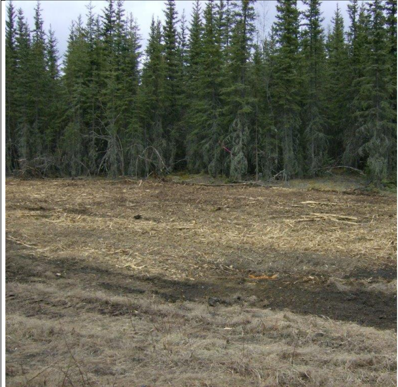
Figure 1.22 Temporary soil stabilization during construction using brush mulch consisting of hydro-ax slash.
