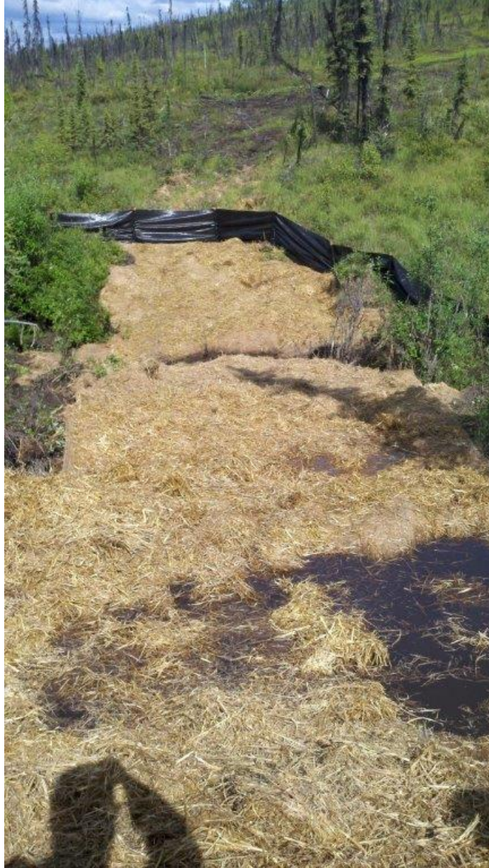
Figure 1.24 Trail rehabilitation near stream crossing using straw mulch, rolled erosion control products (erosion control blanket), perimeter sediment control (silt fence), and seeding with “rehabilitation seed mix.”
