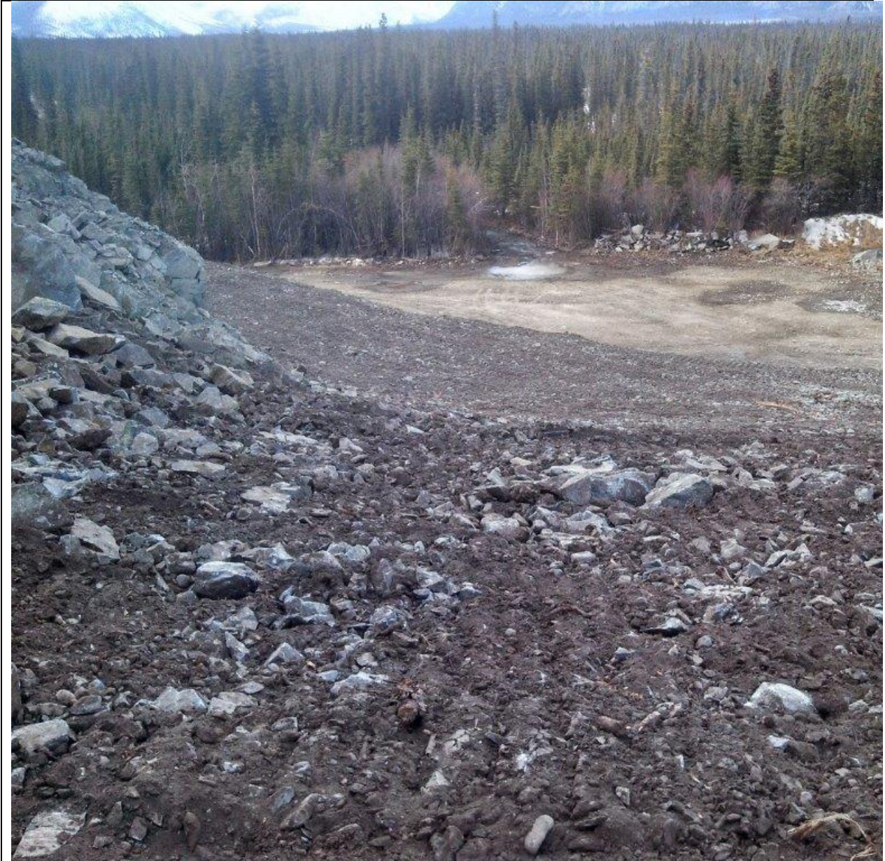
Figure 1.16 Quarry reclamation along Tok Cutoff. Low erodible material with recovered growth media, surface roughening (track walked) prior to application of seed and mulch.
