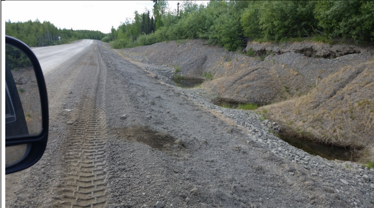
Figure 1.5 Note lack of vegetation on embankment slope, some dead grass. This is rock riprap ditch with planned retention ponds, but slope of lobes has dead grass.
