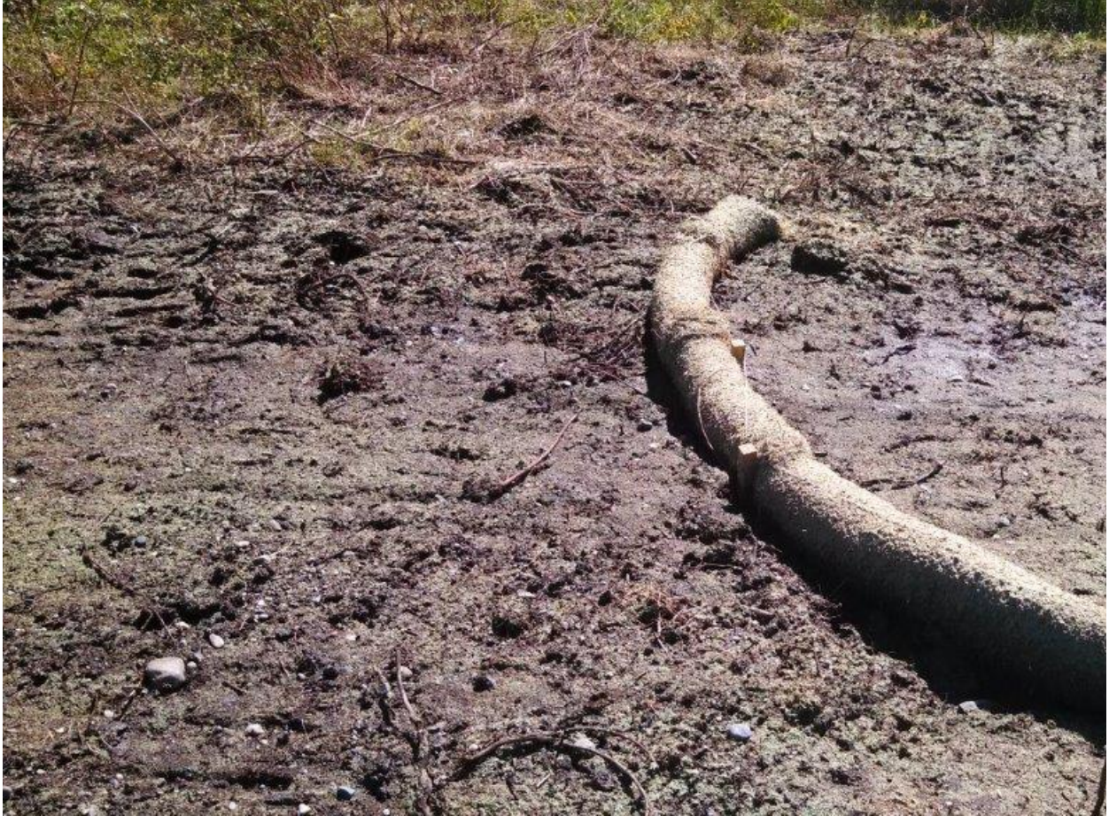
Figure 1.20 Utility line construction showing fiber roll used as velocity dissipation device and hydromulch/seed.
