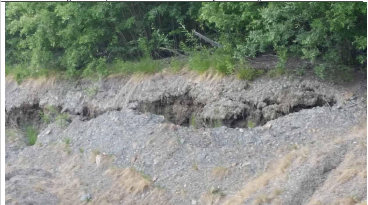
Figure 1.4 Slope failure. Could be permafrost or engineering failure, but note lack of revegetation on slope contrasted with lush growth above the cut.
