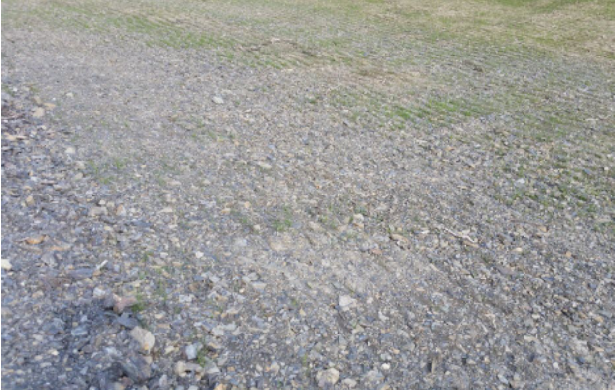
Figure 1.7a (Next 3 photos) MP 100 Elliott Highway, no record of when work was done, seems recent. Tracked.
