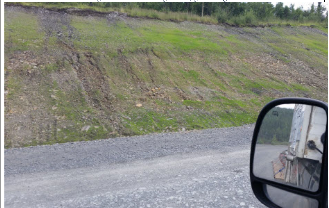
Figure 1.10 Note slope erosion. This is on left/west side MP 108–109. Recent project.
