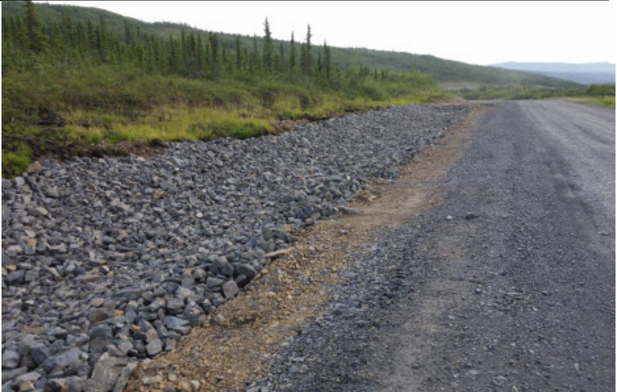
Figure 1.8a MP 108, project opened October 2014, so work was done in 2015 and maybe 2016; riprap in ditch. Upslope side, presumably with organic soils, has grass; roadside, all mineral soils, has no grass.
