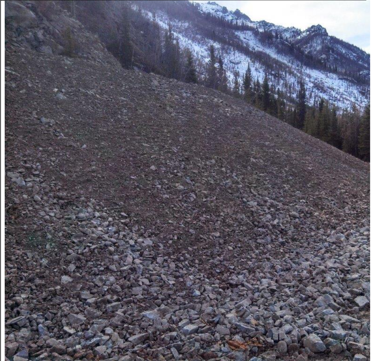
Figure 1.15 Final slope stabilization at a quarry near Tok, Alaska. Low erodible material with surface roughening (track walked).
