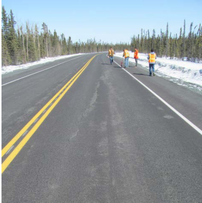
Figure 3.4 Cracking area 3a
