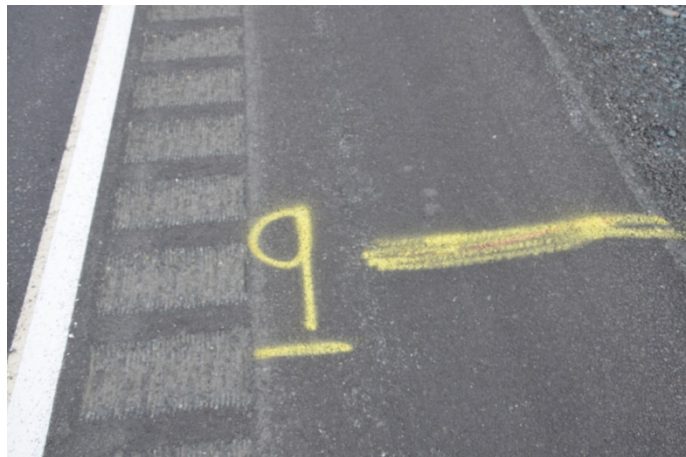
Figure 3.29 G50/50 and G100/100 (sections 9 and 10) no new crack
