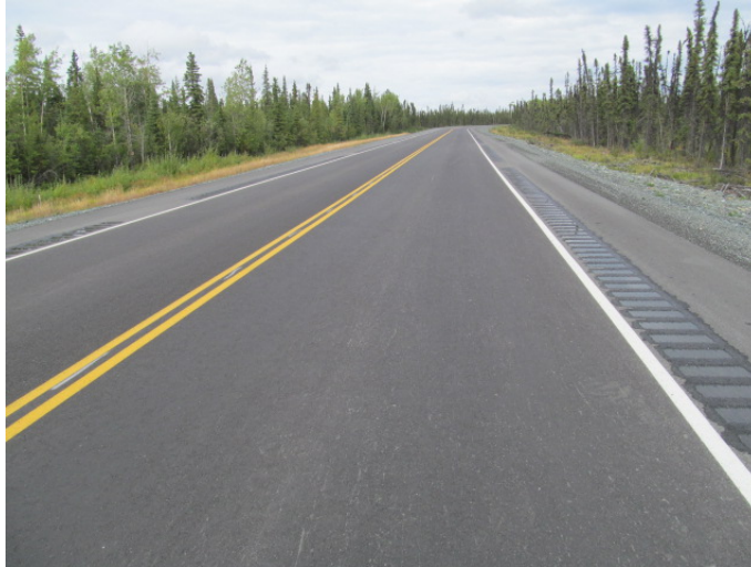
Figure 3.20 G^4 test section (reinforced with 300 feet of G^4 paving interlayer in the right lane in area 2, no visible cracks)
