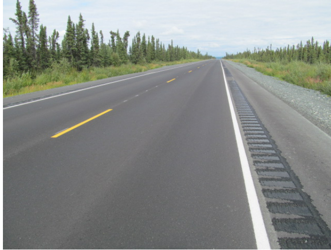
Figure 3.22 G100/100 test section (reinforced with 300 feet G100/100 in the left lane in area 10, no visible cracks present)
