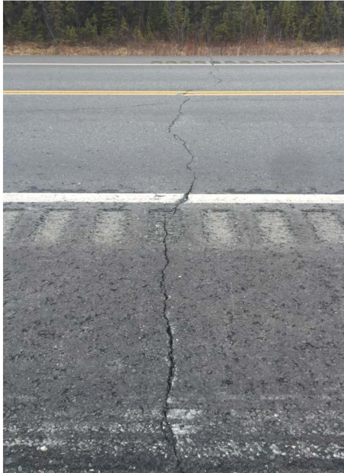
Figure 3.38 Evolution of a transverse crack from minor to major in G 4 test section
