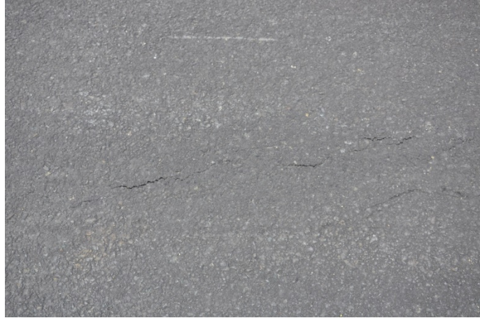
Figure 3.28 G 4 section (area 2) new minor crack
