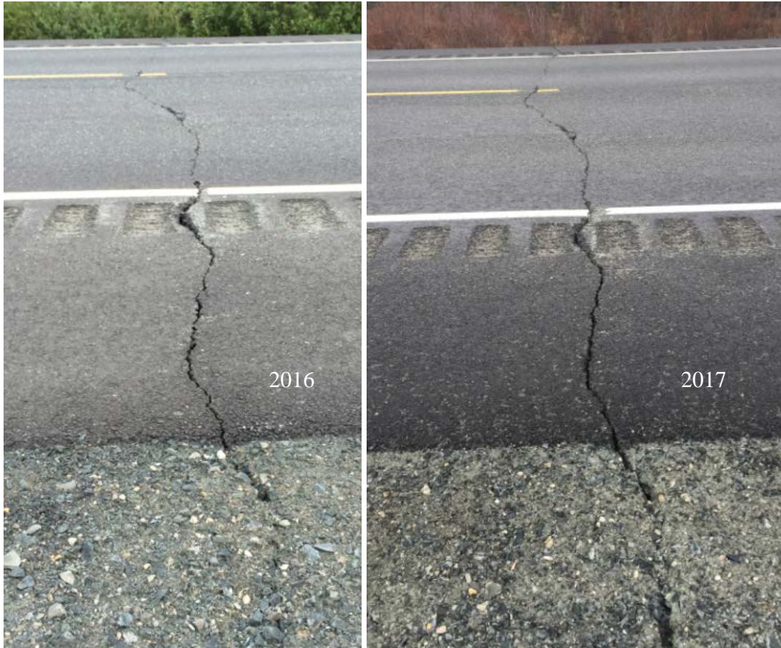
Figure 3.39 A transverse crack in G50/50 section
