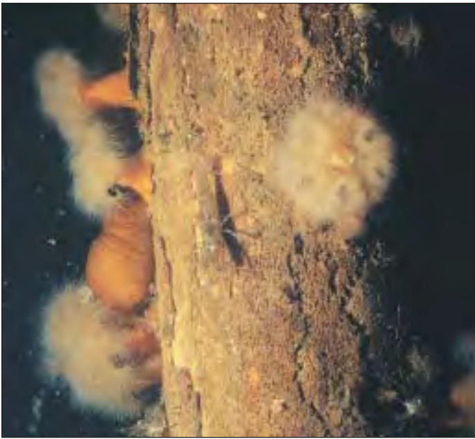
The untreated piling were deteriorating and did not support a vibrant fouling community
