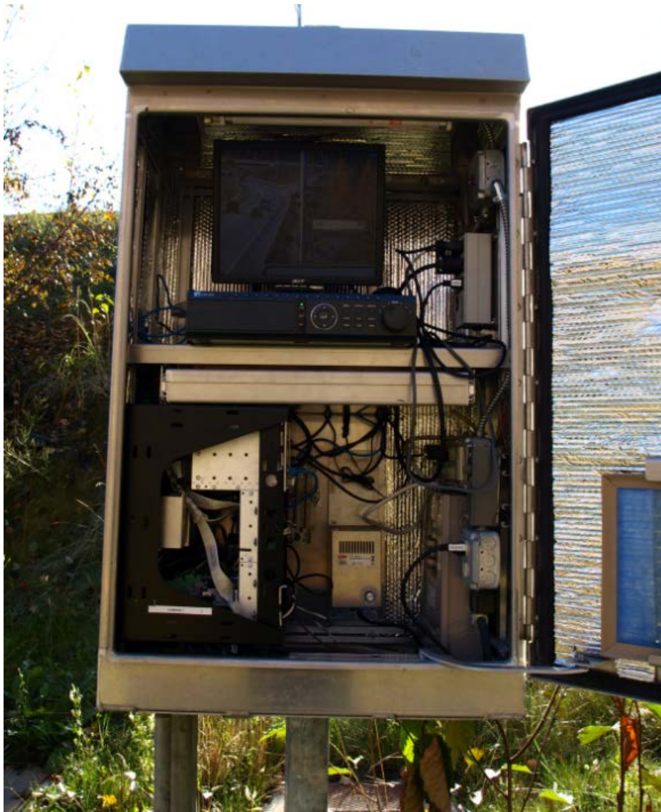
Figure 5 Overheight Detection System Controller Cabinet
