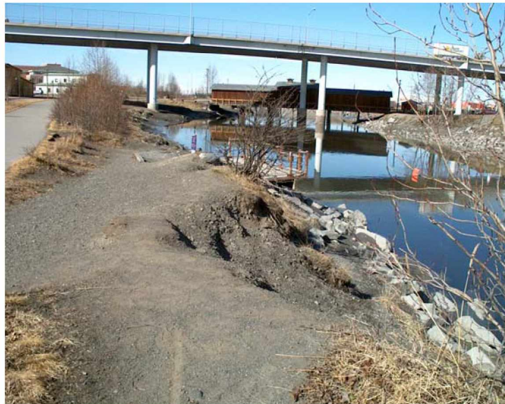
Figure 14: Bank Erosion, Ship Creek, 2003.
