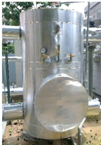
Fig. 2.5 Hot water storage tank
