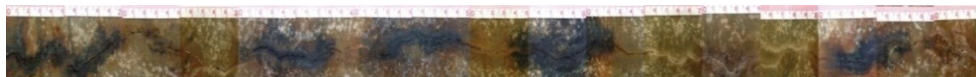
(c) Spatial variability in the surface crack widths and photos of the corrosion cracking
