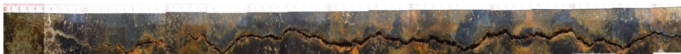
(c) Spatial variability in the surface crack widths and photos of the corrosion cracking
