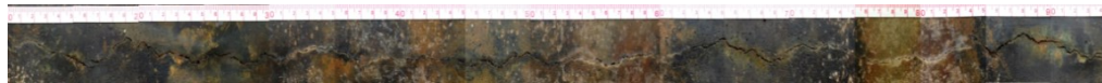
(c) Spatial variability in the surface crack widths and photos of the corrosion cracking
