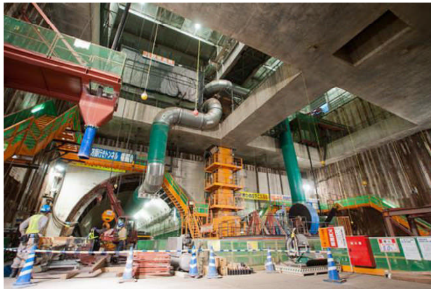
Figure 4.4. Entrance of tunneling route down through the shaft below the shin-Yokohama area (reproduced from the http://radiate.jp/20111111/kouza34/# )
