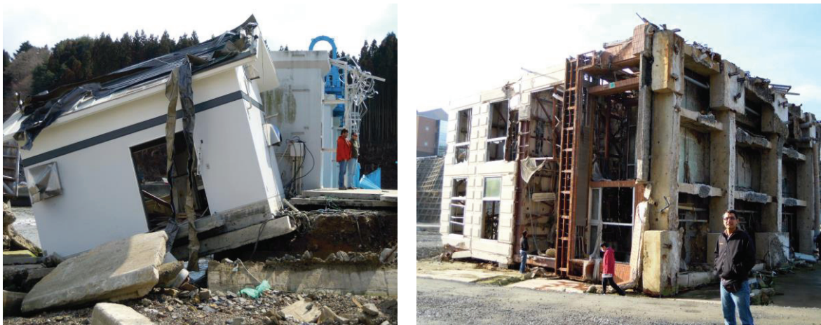
Figure 10. Effects of 2011 Japan Tsunami. Left: Scour in coastal facilities at Minami Sanriku. Right: Four-story building turned down at Onagawa.
