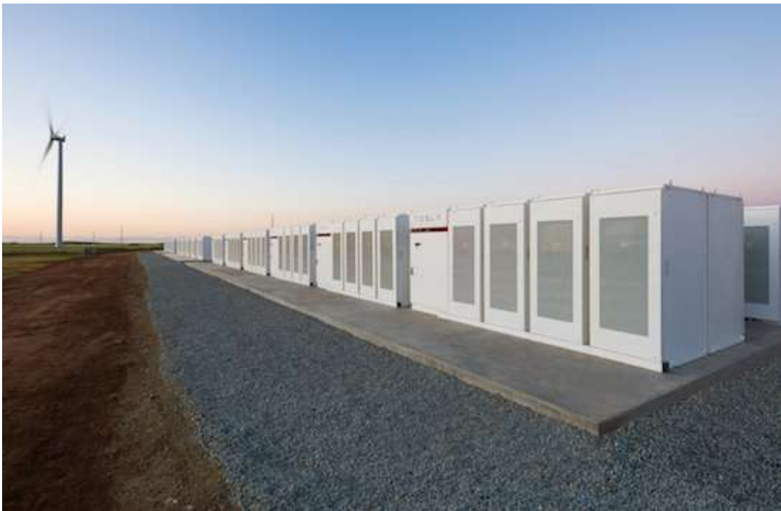
Figure 7: 100MW Tesla Battery Pack in SA
