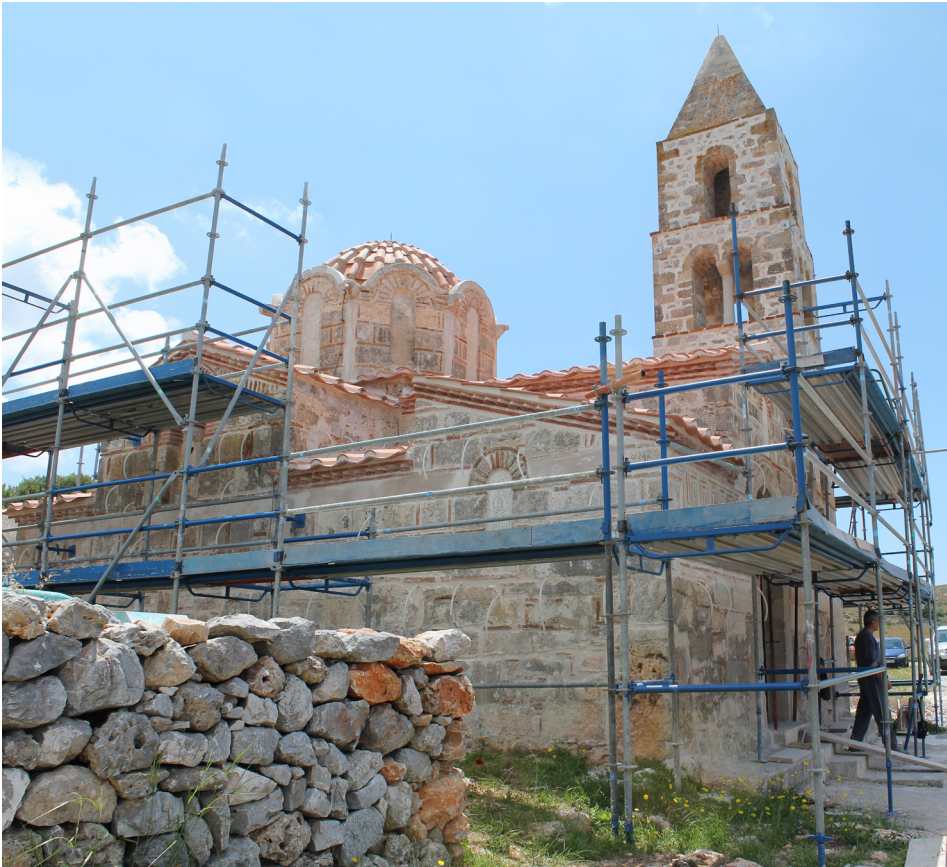
Figure 10. The 12 th -century church of Agios Nikolaos undergoing renovation by the regional archaeological authority (May 2014). The renovation was completed soon after this photo was taken.
