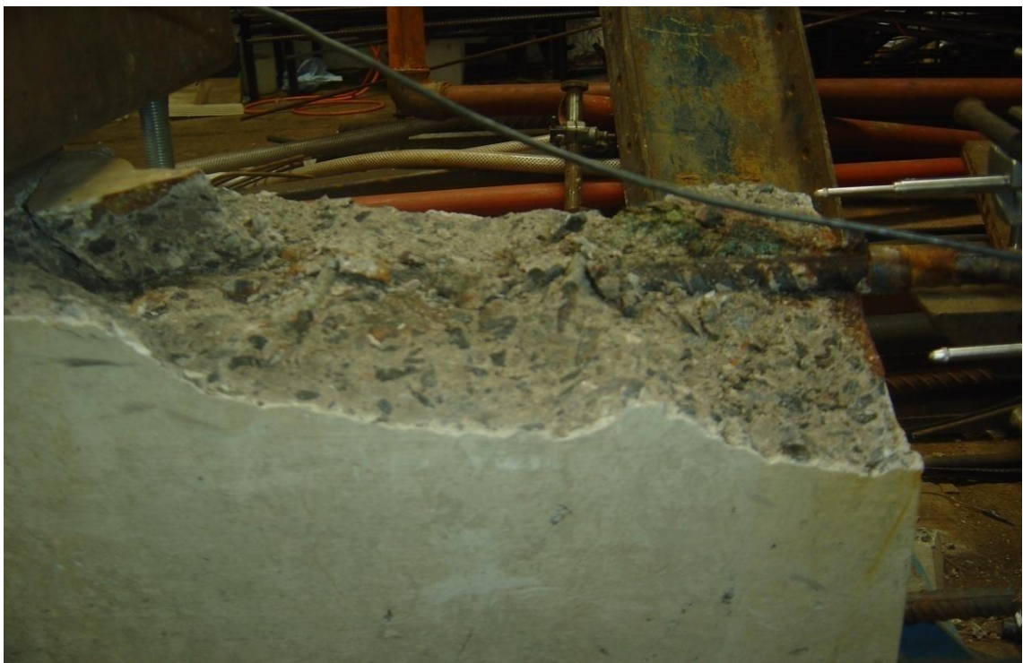
Figure 5.19: Splitting failure on centre bar location
