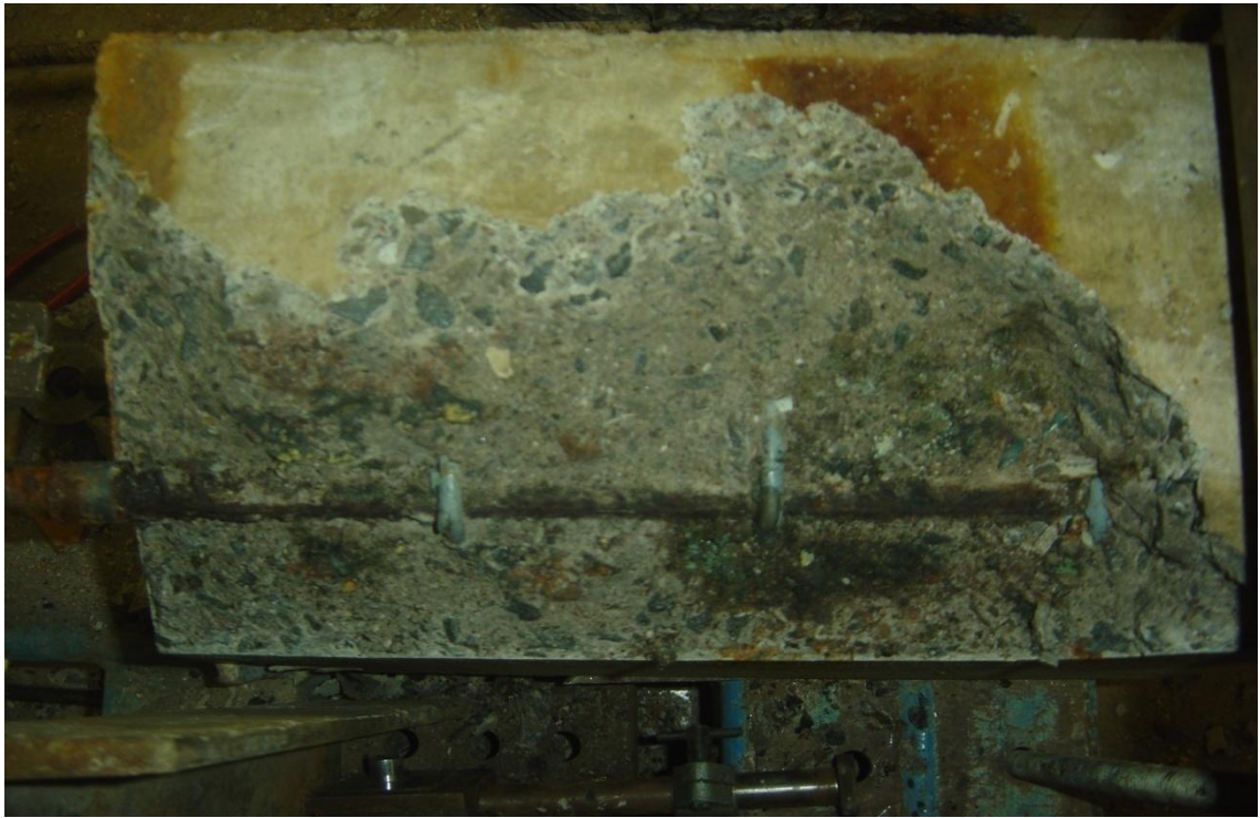
Figure 5.20: Splitting failure on corner bar location
