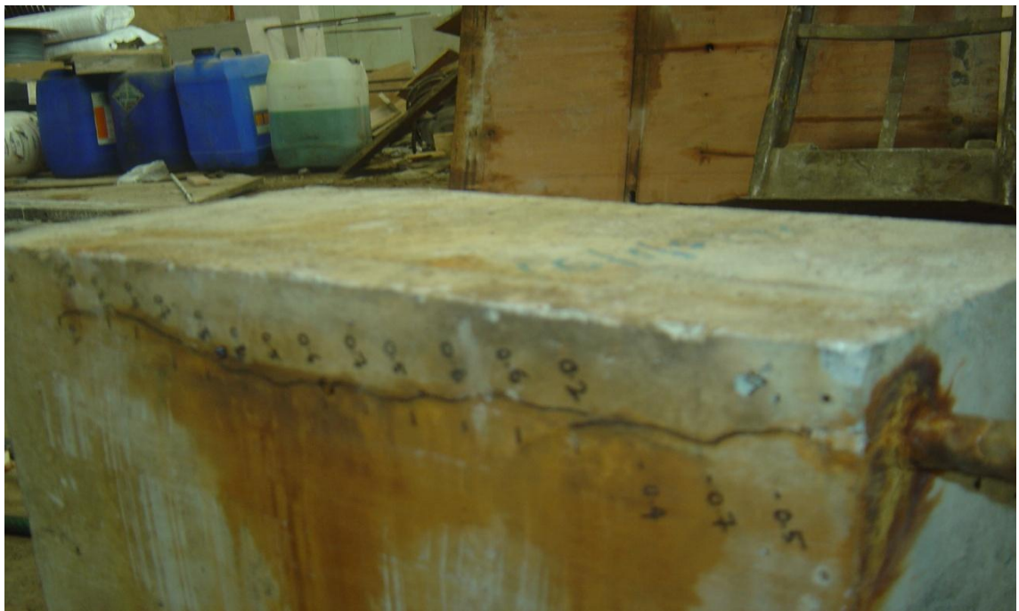
Figure 5.11: Longitudinal surface crack on corner bar location
