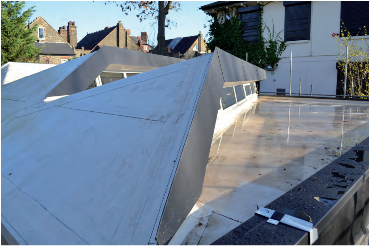
Fig. 12 Roof after rain shower
