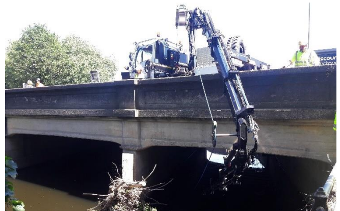
Figure 3: BridgeCat vehicle taking sonar scans before repair
