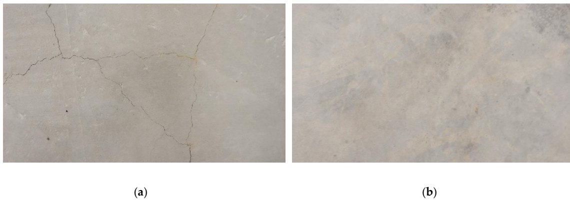
Figure 3. Representative images of (a) cracked concrete and (b) sound concrete.
