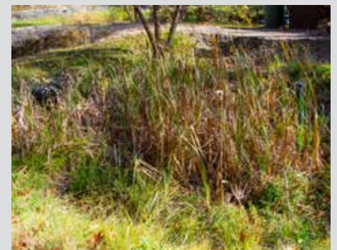
Un-maintained gravel wetland at the field site reflects the standard of practice and is an excellent opportunity for research to support operations and maintenance for this system.
