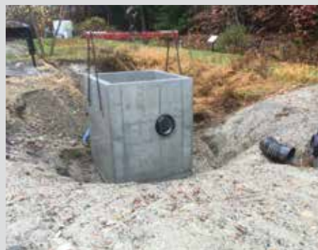
Three new manufactured systems were installed at the UNH Stormwater Center’s field site in fall of 2019.
