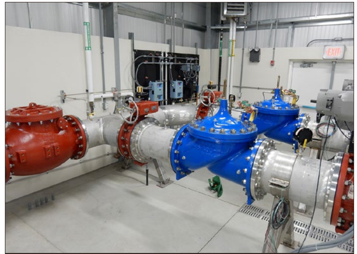
Unalaska Pyramid Water Treatment Plant, Eklutna Services, Inc.
