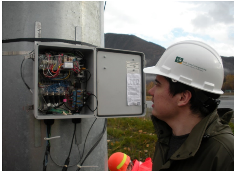
Figure 4.11: Completed Data-acquisition System at Peter's Creek HMLP
