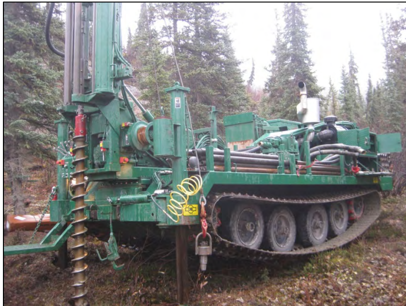
Figure B-1. Typical rig set-up for hollow-stem auger, with the CME 850X track-mounted drill. Photograph taken while drilling TH12-9000. (Photograph by M. Darrow)
