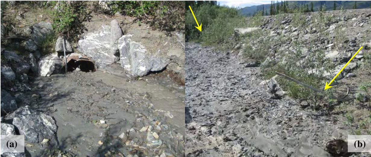
Figure 4. Evidence of sedimentation from the outflow of FDL-A. (a) A culvert inlet nearly buried with recent deposition. (b) A second culvert inlet is already buried by the sediment (see right arrow). The location of the culvert in (a) is indicated with the arrow to the left in (b). (Photographs by M. Darrow)
