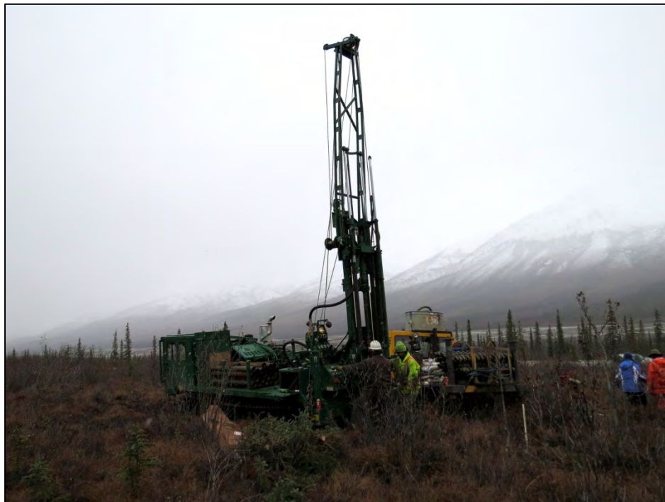
Figure B-4. Location of TH12-9002. View is to the southwest, with the Dalton Highway visible in the middle-right of the figure. (Photograph courtesy of M. Carew)
