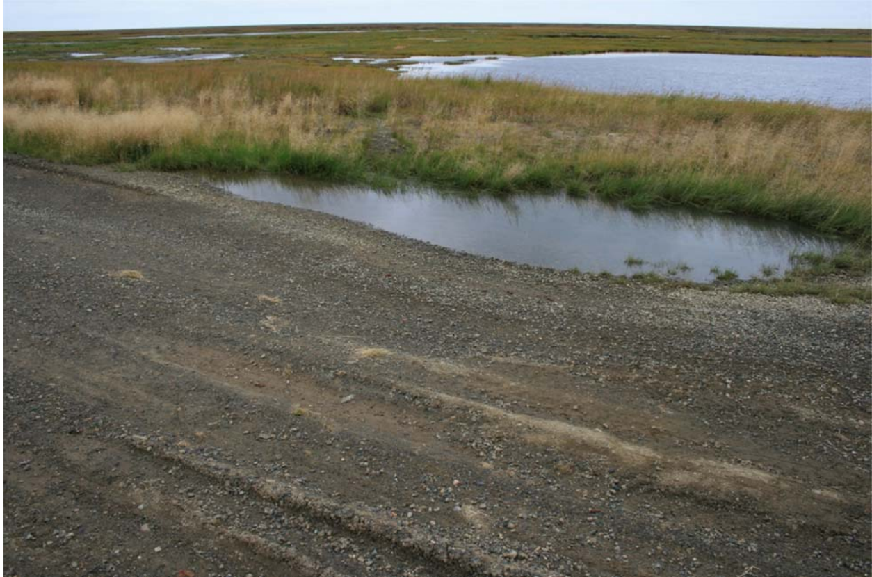
Figure 5: Ruts caused from melting permafrost on northern end of runway
