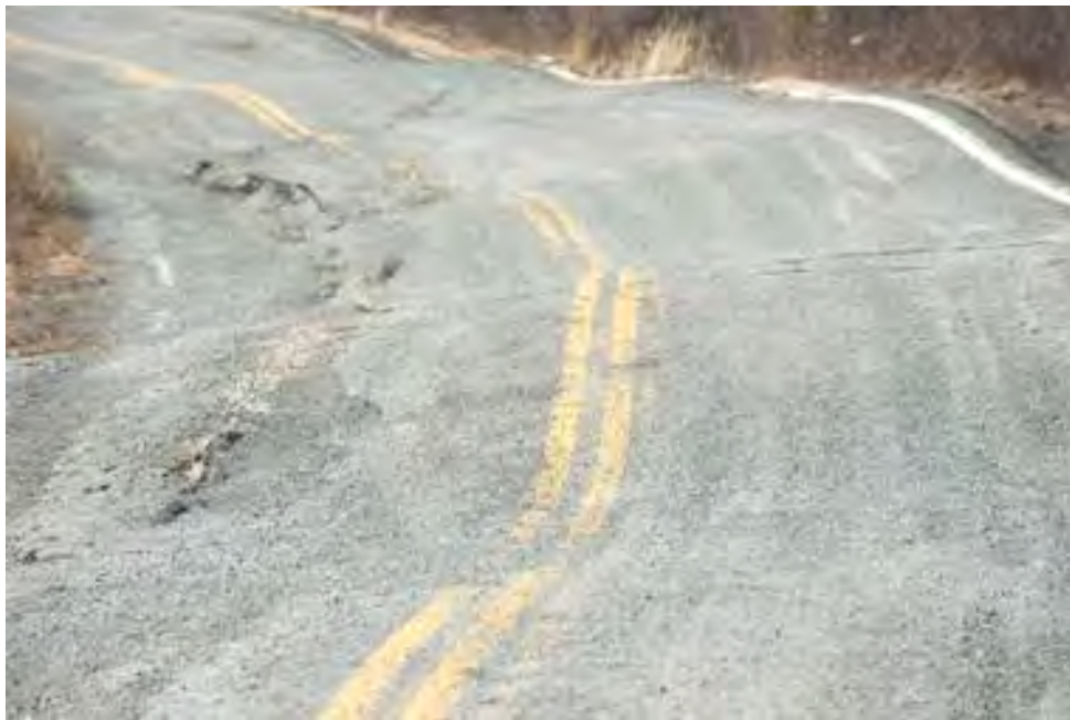
Figure 24 - Example of a permafrost-damaged road in Alaska.
