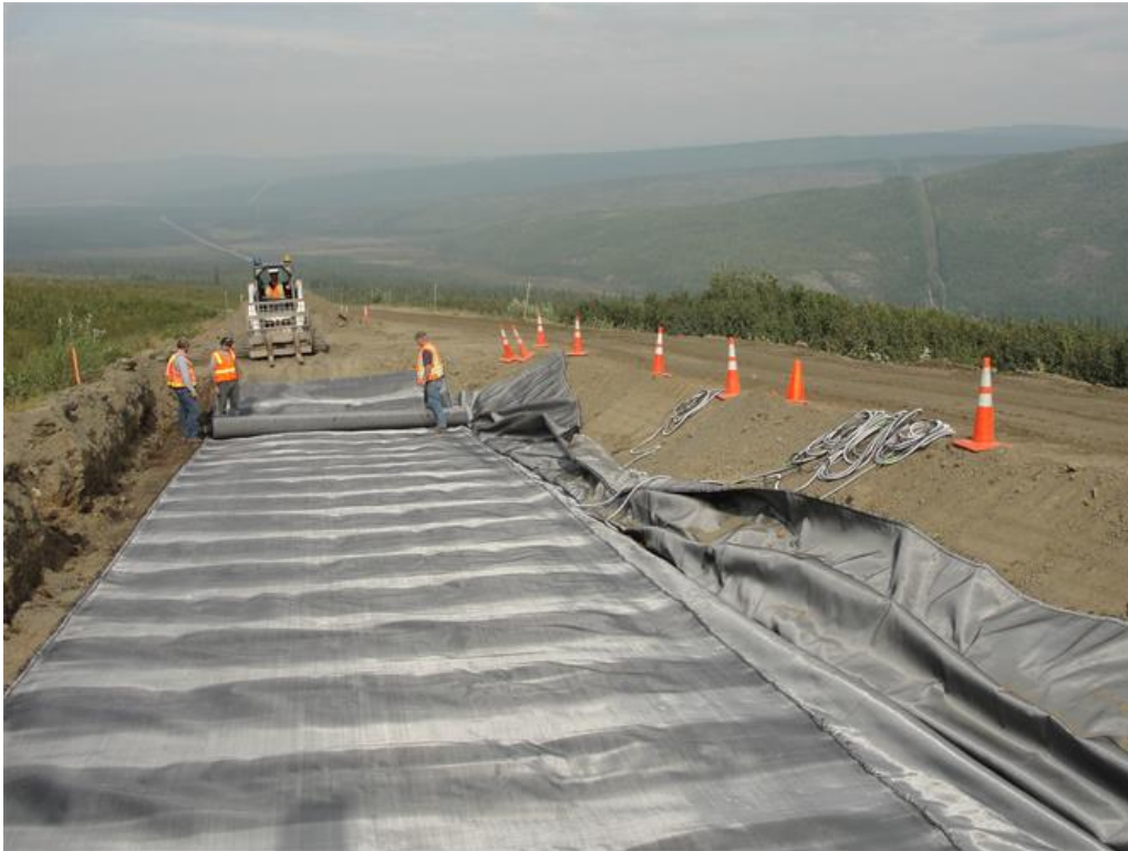
Figure 37. Installation of the first layer of wicking fabric on the west side of the road
