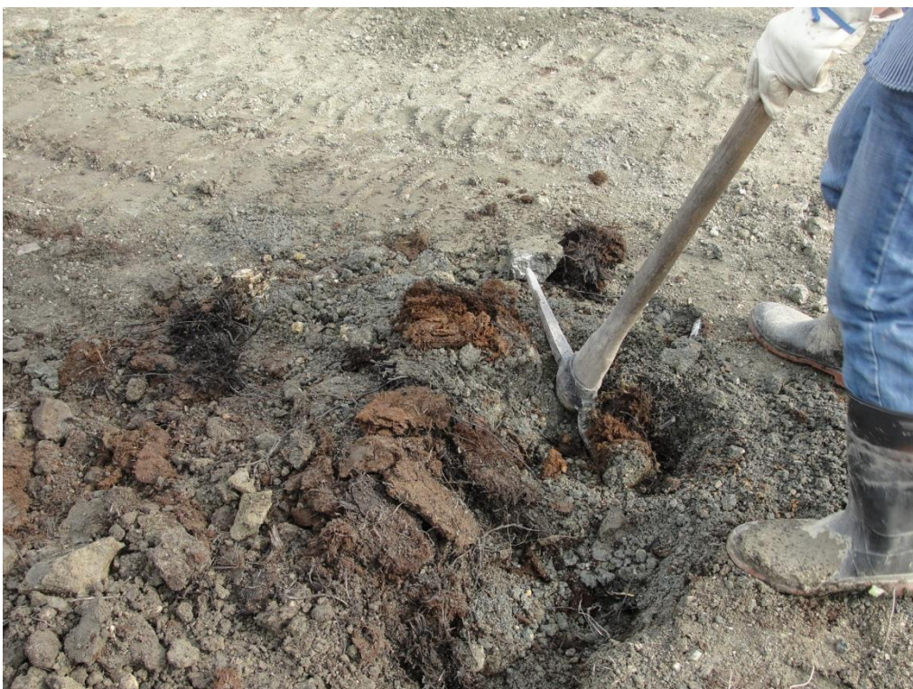
Figure 33. Degraded vegetation layer found on the bottom of the excavation
