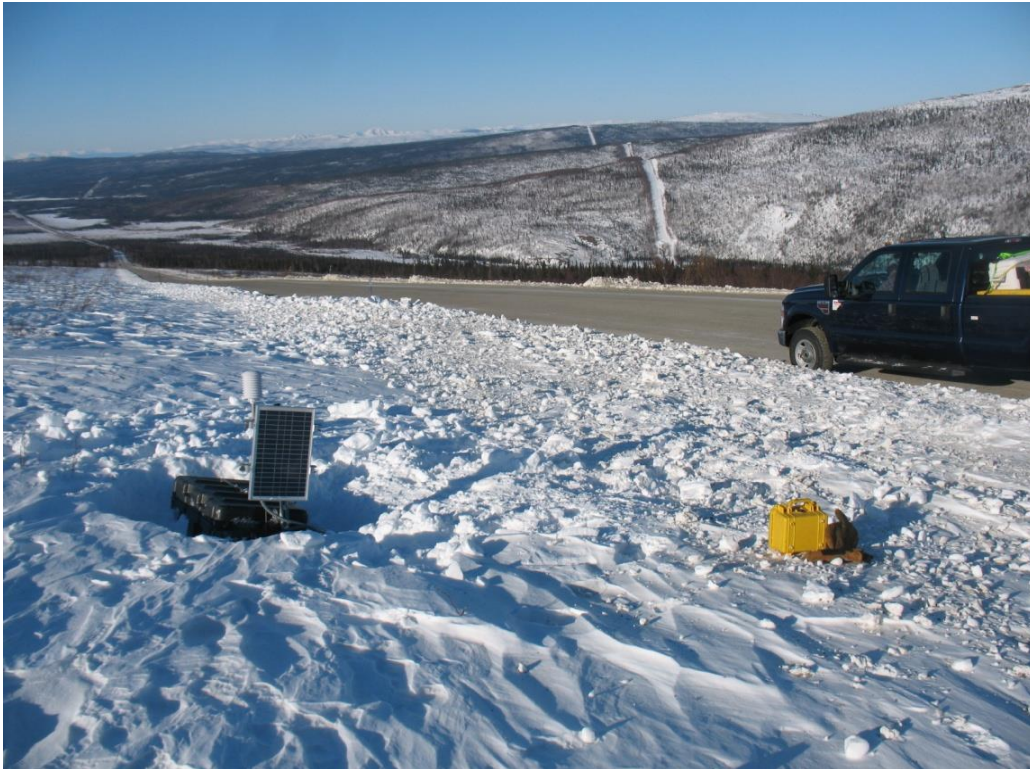
Figure 55. Data collection box after installation of the solar panel
