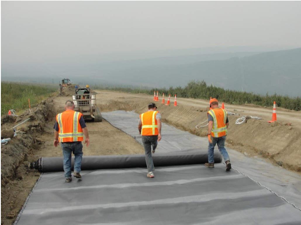
Figure 40. Installation of the second layer of wicking fabric on the west side of the road
