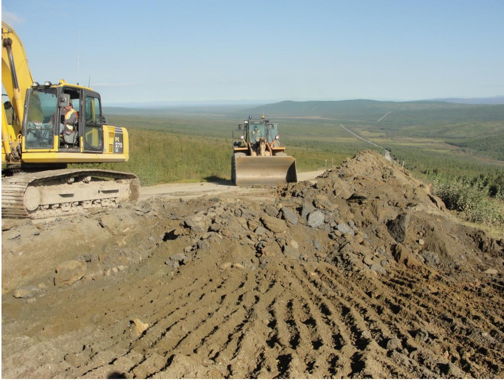
Figure 21. Excavation of the lane on the east side of road (looking north)
