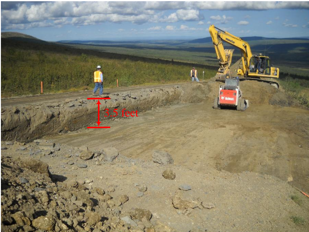
Figure 22. Excavation of the lane on the east half side of road (looking north)
