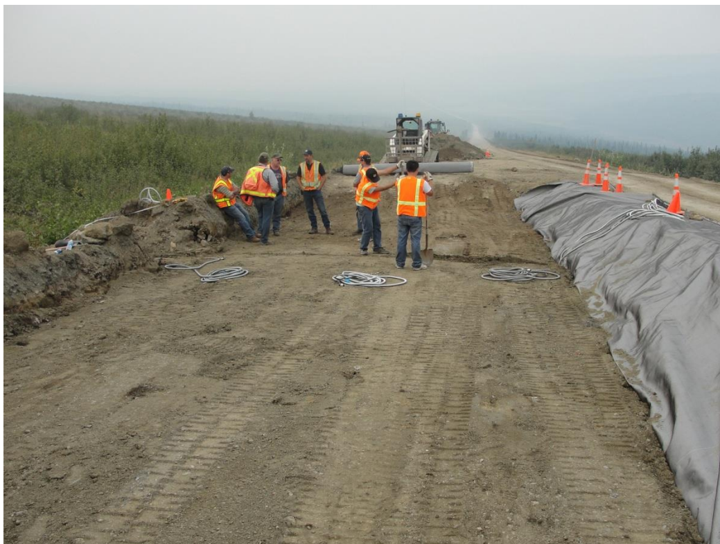
Figure 39. After installation of the first layer of wicking fabric on the west side of the road
