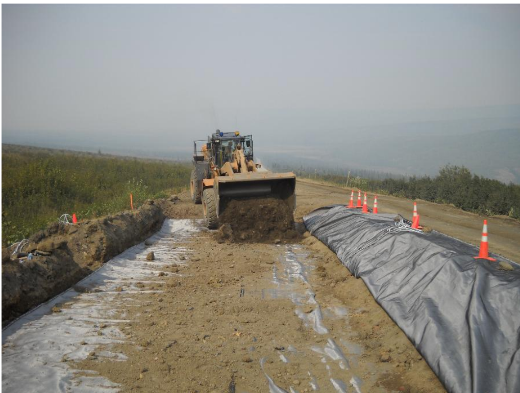
Figure 38. After installation of the first layer of wicking fabric on the west side of the road
