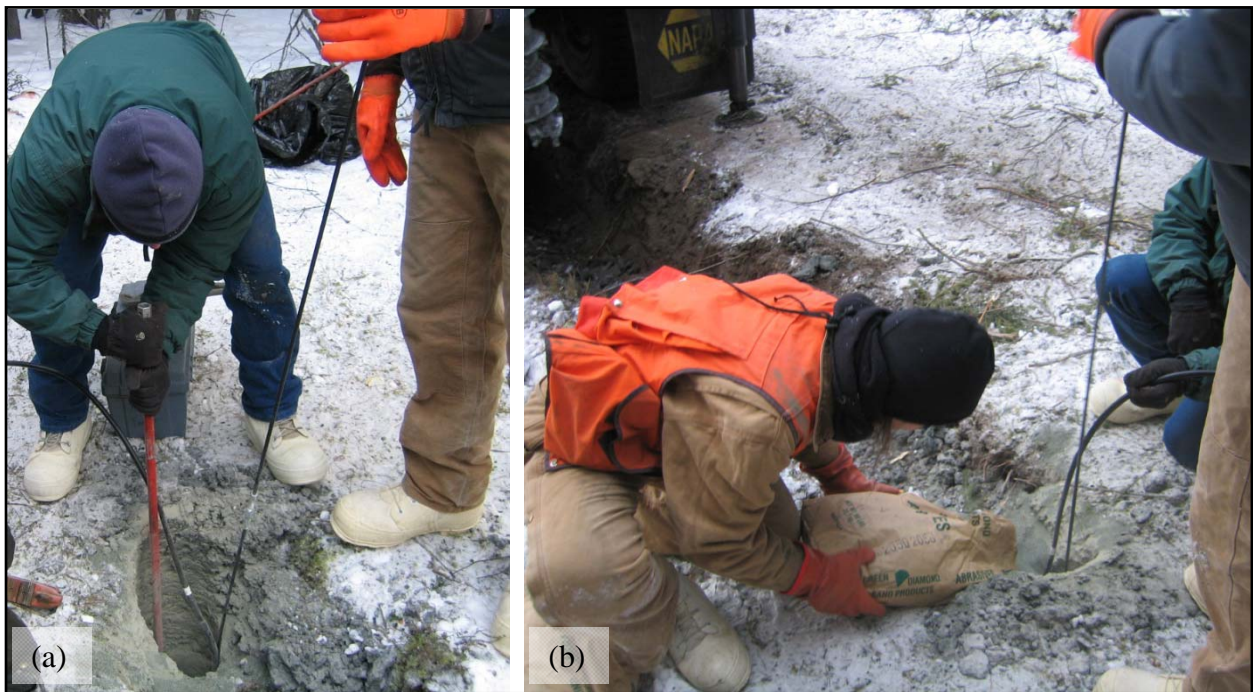
Figure 2.9. Installing a thermistor string: (a) backing off the steel rod (red in color); (b) backfilling and tamping the test hole.
