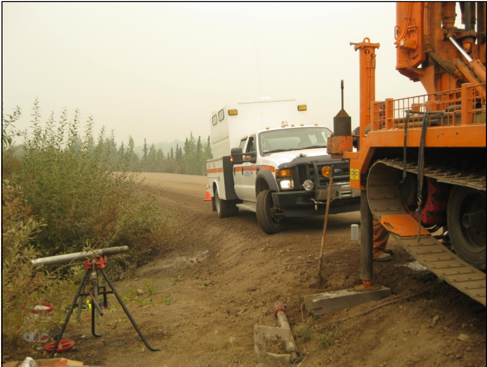
Figure 3.7. Drilling TH09-1403 on the Dalton Highway shoulder. The apparent embankment height in this photograph is about three feet; the embankment thickness as drilled is approximately 10 feet.
