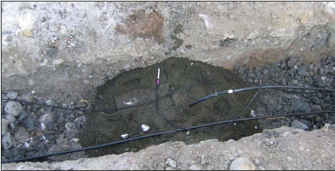
Figure 2.10. Thermistor cables at the bottom of the trench at the TH08-1654 location, prior to backfilling. Note the CS107 sensor laying on the sandy backfill. Its exact placement occurred during the final backfilling of the trench.
