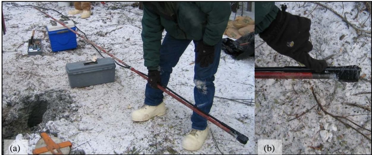
Figure 2.8. Staging a thermistor for installation: (a) extending the thermistor string along the steel rod; (b) thermistor end attached to the “sacrificial” coupler.
