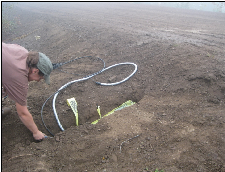
Figure 3.8. Excavating a burial trench by hand through the embankment and side slope. In this photograph, the trench in the shoulder already was backfilled. The thermistor cable (black) and CS107 cable (in flexible conduit) were placed at the bottom of the trench below caution tape.
