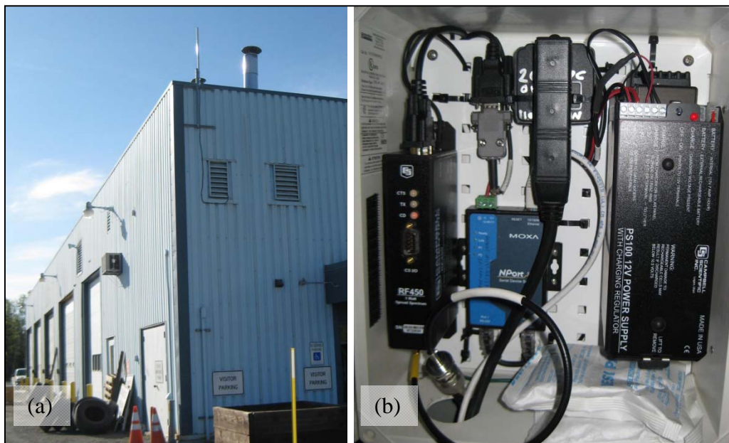
Figure 2.15. Telemetry components at the Tazlina M&O station: a) 900 MHz omni directional antenna mounted to the outside of the building; b) enclosure containing RF450 900MHz 1W spread spectrum radio, Moxa portserver, and 12 Vdc power supply with charging regulator and 7 Amp-Hr sealed rechargeable battery. The enclosure is mounted to a wall in the corner room on the second floor the building (the room contains the grate through which the antenna cable runs in (a)).
