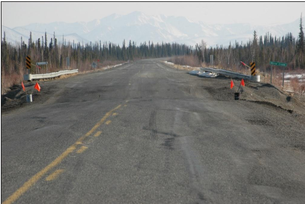
Figure 2. Transverse depressions in the surface of the Alaska Highway due to permafrost degradation. (Photography courtesy of D. Fortier)
