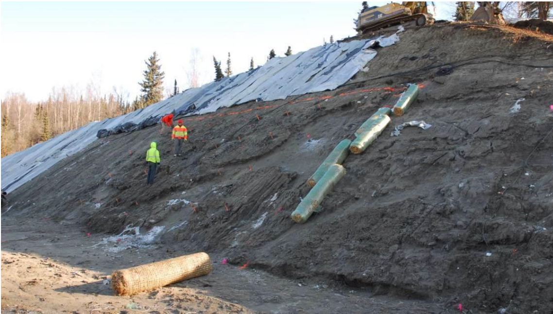
Figure 4.7 Cut slope erosion during construction
