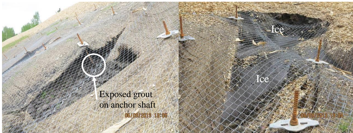
Figure 6.3 Close views showing exposure of soil anchor grout (left) and portion of massive ice feature under Tecco-mesh (right)
