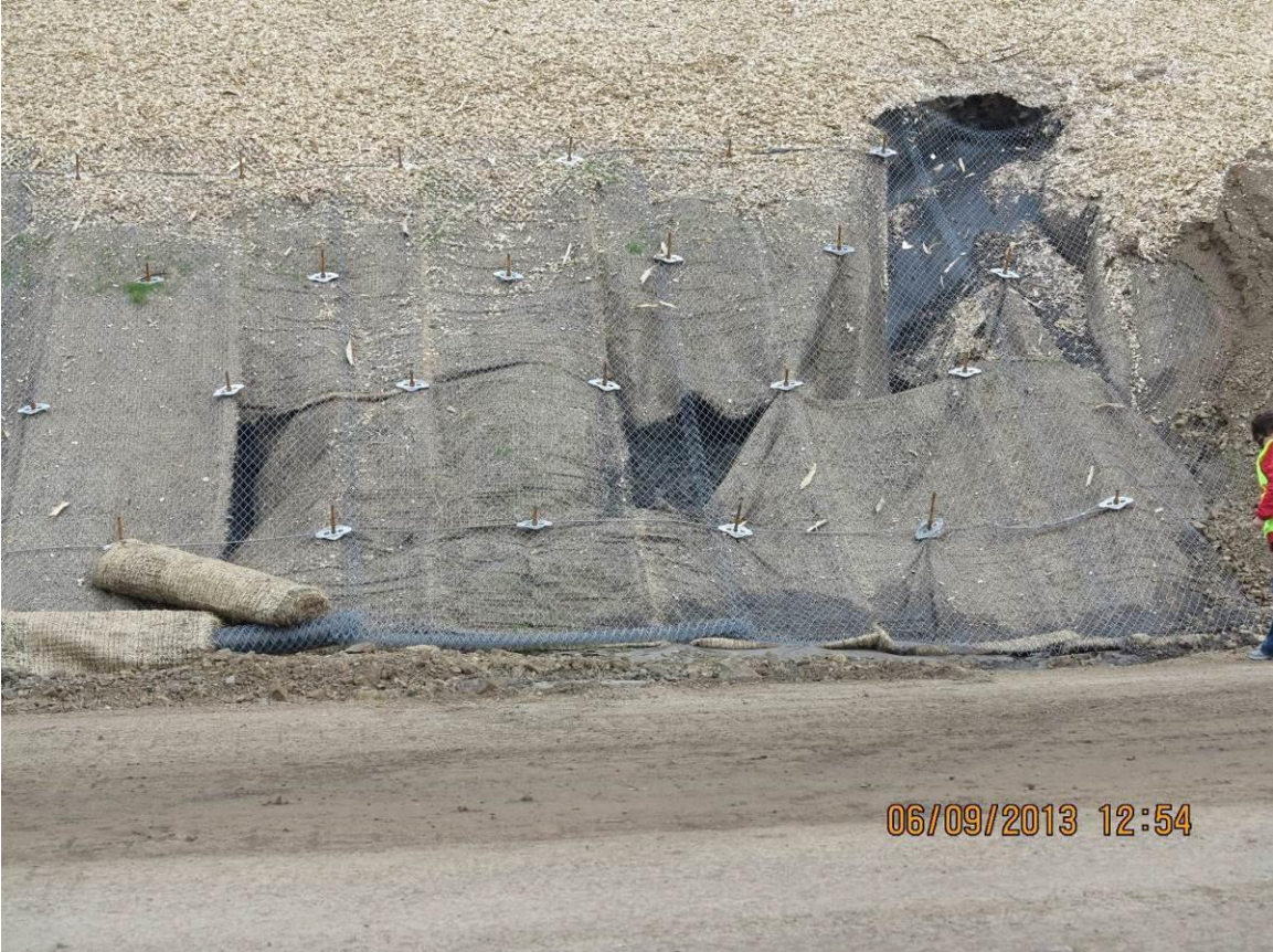
Figure 6.2 Close view of failure within the Tecco-mesh section
