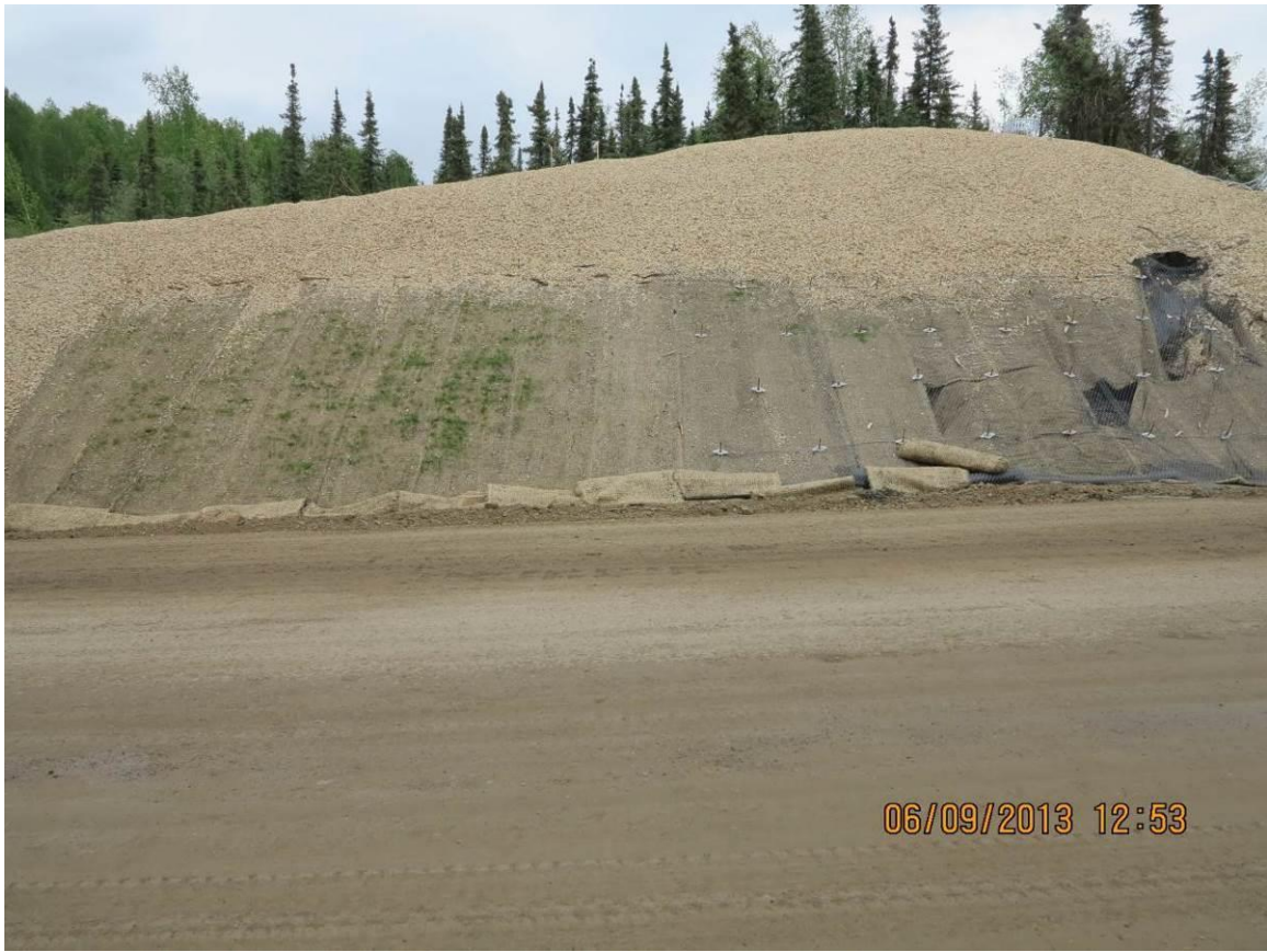
Figure 6.4 Surface protection matting in area showing no grass growth is not in direct contact with ground surface
