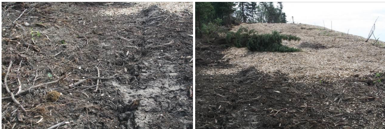
Figure 6.9 Start of thaw related damage at top of Experimental Feature cut slope
