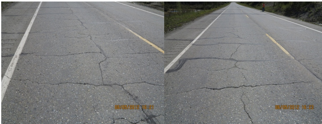
Figure III.8 Lessor thermal cracks—moderate (note some very old sealant in left photo)
