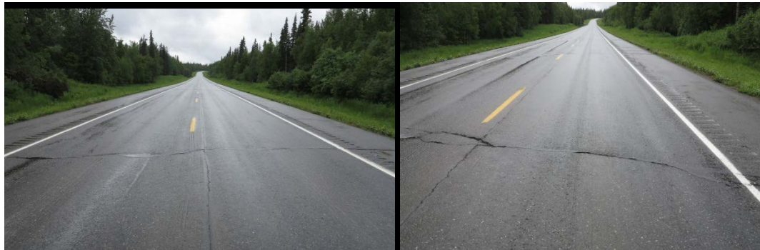
Figure V.15 Severe major transverse cracks with little influence on pavement performance beyond crack edges (very common)
