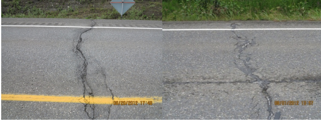
Figure III.5 Examples of spalled zones along major transverse thermal cracks
