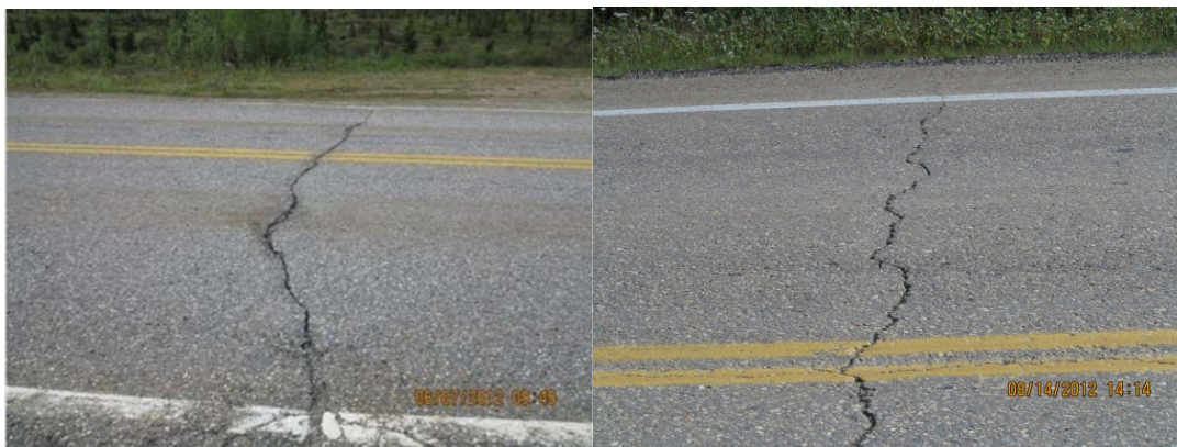
Figure III.1 Regular appearance of major transverse thermal cracks
