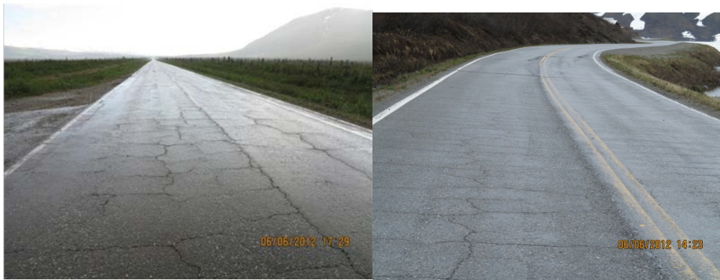
Figure III.9 Lessor thermal cracks—severe (no sealant)
