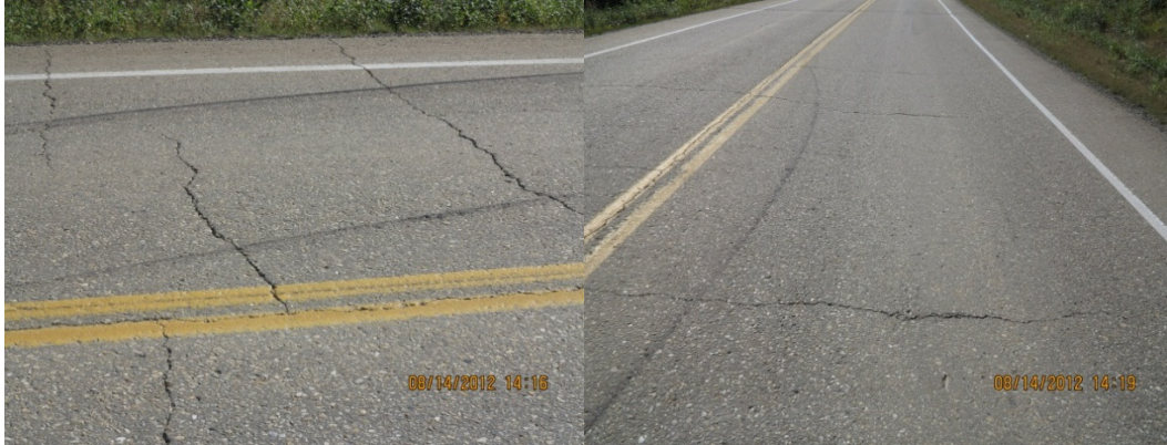
Figure III.7 Lessor thermal cracking—slight w/ cracks wider than 1/8 inch
