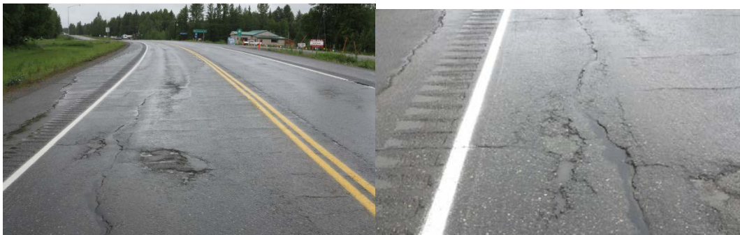
Figure V.17 Examples of pavement delamination damage accentuated at crack locations
