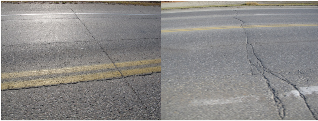
Figure VI.1 25+ year old major transverse thermal cracks, precut (left) natural (right)
