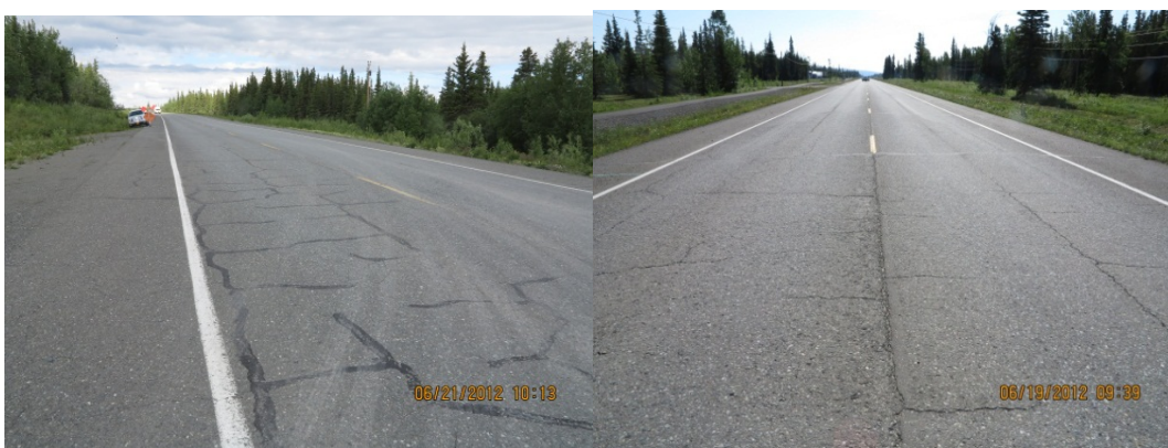
Figure III.6 Lessor thermal cracking—slight (note sealing in left photo)
