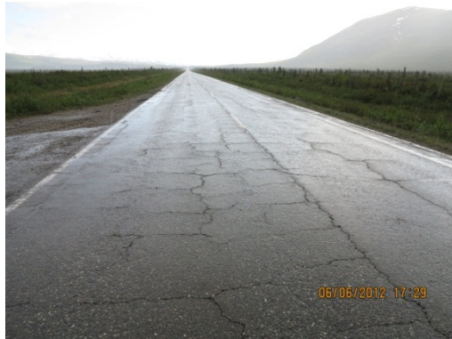
Figure I.1 Example of lesser thermal cracking
