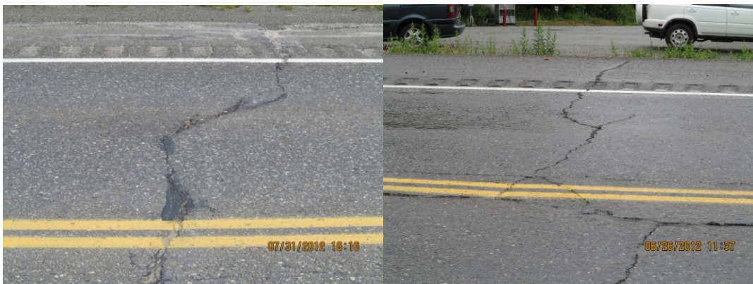
Figure III.3 Examples of crooked major transverse thermal cracks
