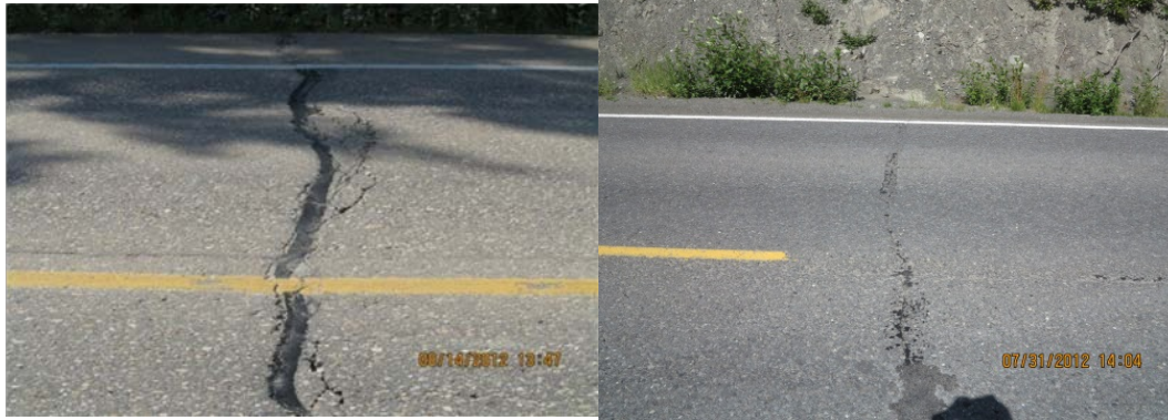
Figure III.2 Major transverse thermal cracks with new sealant (left) and old sealant (right)
