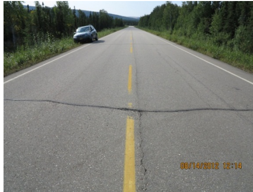
Figure I.2 Example of Major transverse thermal crack
