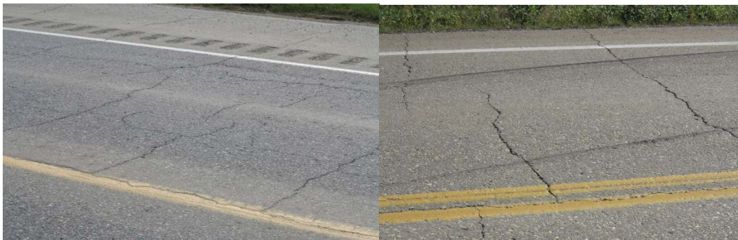
Figure V.14 Lesser thermal cracks showing same performance in wheel path and non-wheel path locations (extremely common appearance)
