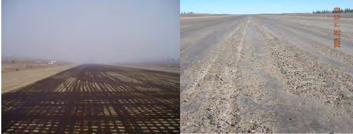
Figure 5.8 improper application (left) and performance (right)
