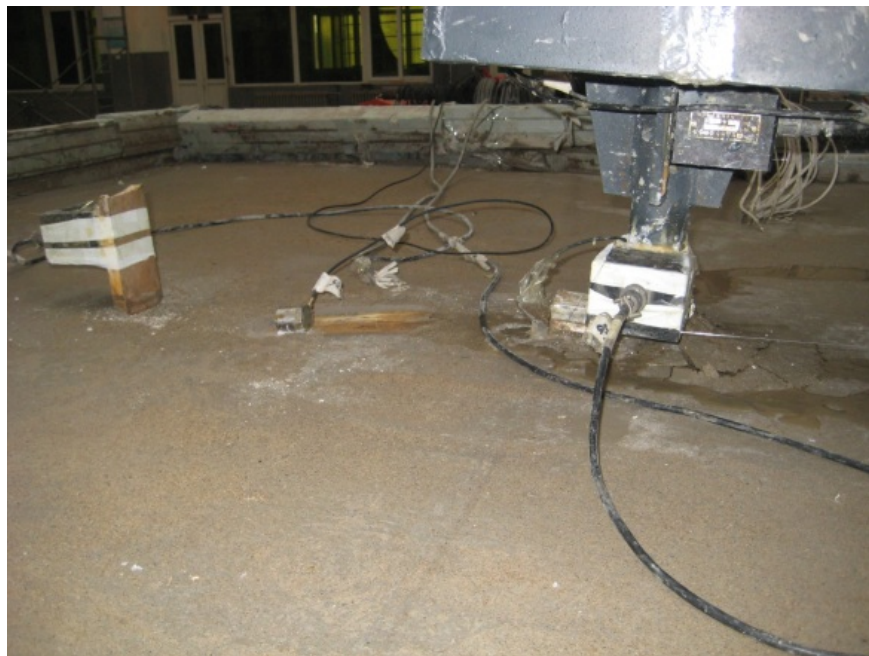
Figure 2.17. Tilted pile head
