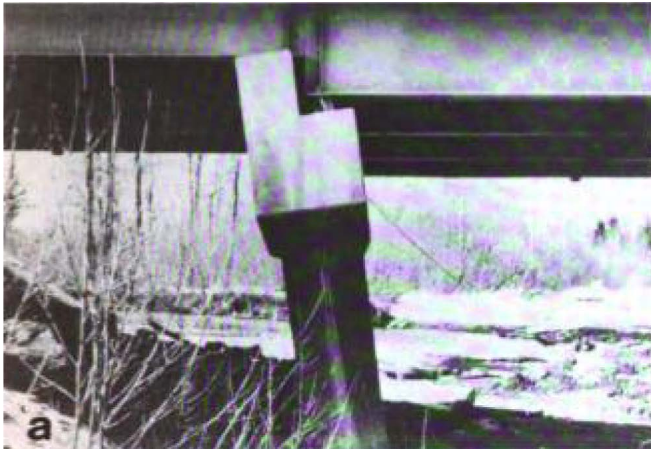
Figure 1.2. Tilted bridge pier due to laterally spreading frozen crust
