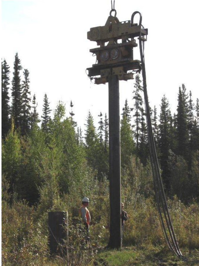
Figure 2.9: Installing a test pile using a vibration head (photo by INE staff).
