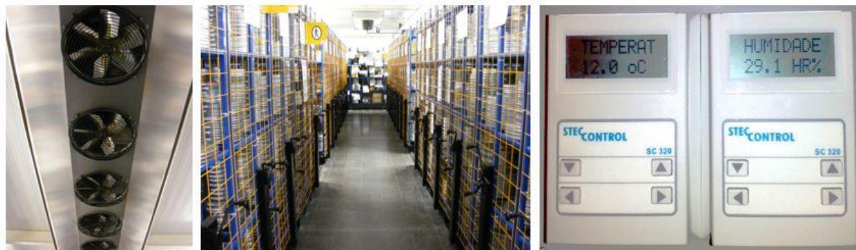
Figure 18 – Cooling air supply (left), interior view (middle), control panels (right) © Teréz Somfai
