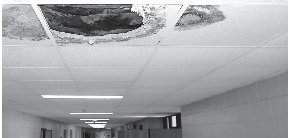
Rain damage stained several tiles and left one nearly 2-foot hole in the ceiling of the Agriculture Building's main hallway Monday. Trashcans and recycling bins were placed under various leaking tiles, which continued to drip into the evening.
