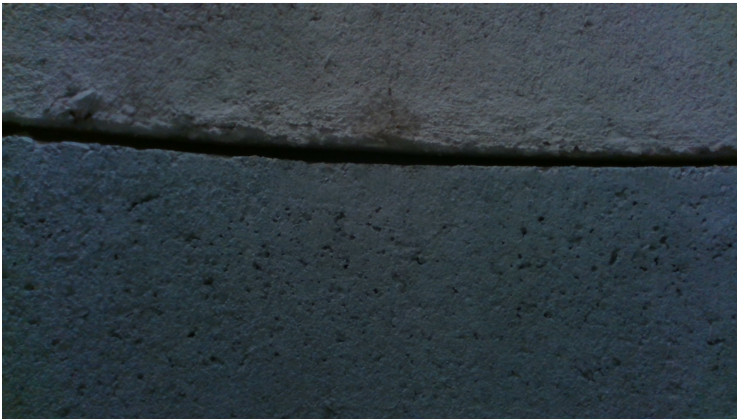
Figure 41: Picture of inner wall of the manhole.
