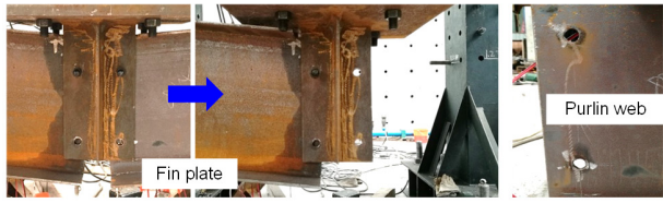
Specimen S2: fracture of bolts on both sides
