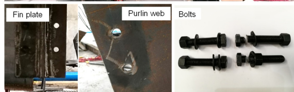
T(R) - Top bolt at RHS fractured
