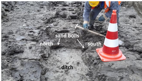
Figure 5 View on the upstream edge of the ditch with sand originating from two sand boils
