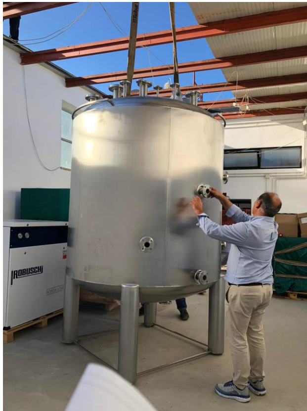
Fig. 113: Fermenter's positioning inside the space dedicated to the indoor pilot plant.
