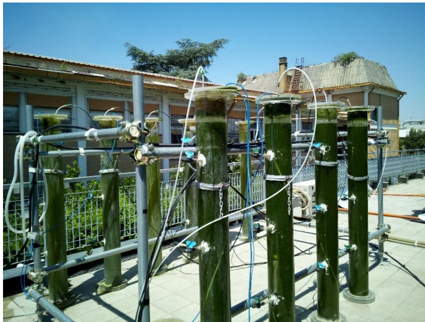
Fig. 43 Working pilot plant installed in Bio-P srl site (N 41°55' 5" E 12°35' 35").
