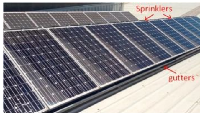
Figure 23. Visual layout of water sprinkler cooling system (Castanheira A., Fernandes J., Branco C., 2018)
