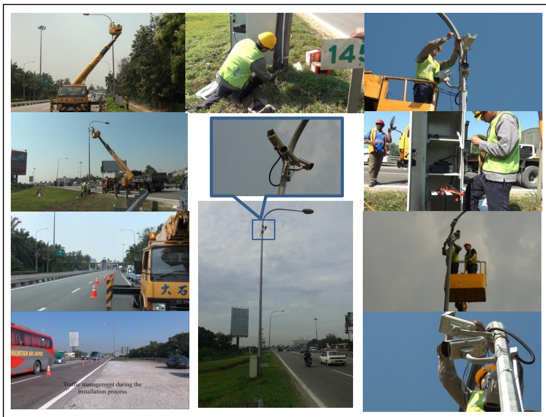
Figure 3.18 Installation process for the CCTV system cameras at Juru and Jawi toll plazas.
