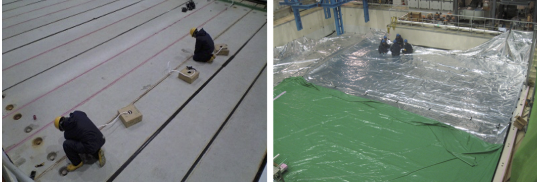
Figure 47: Pictures of the air-tight schemes in the Target Station ground floor. Left: Caulking between the concrete blocks. Right: Air-tight sheet on the concrete blocks.
