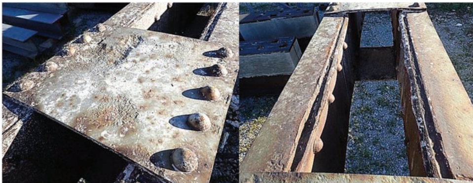
Figure 1.2 View of corrosion damage resulting in section loss and pack rust.
