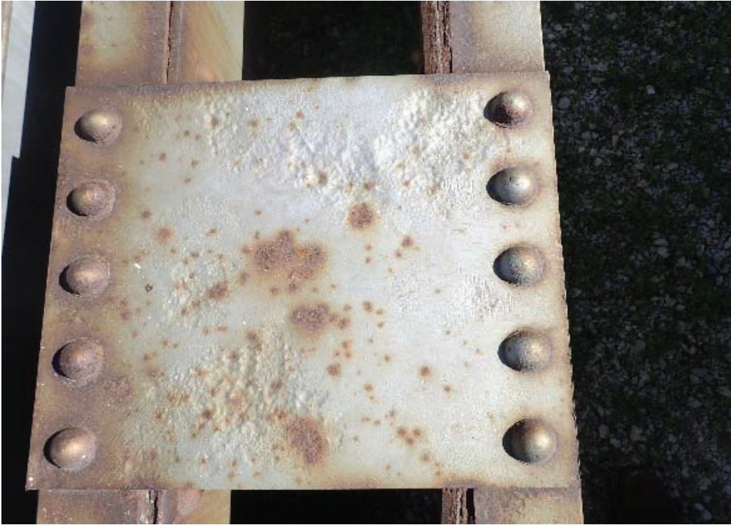
Photo 5: General condition of batten plates
