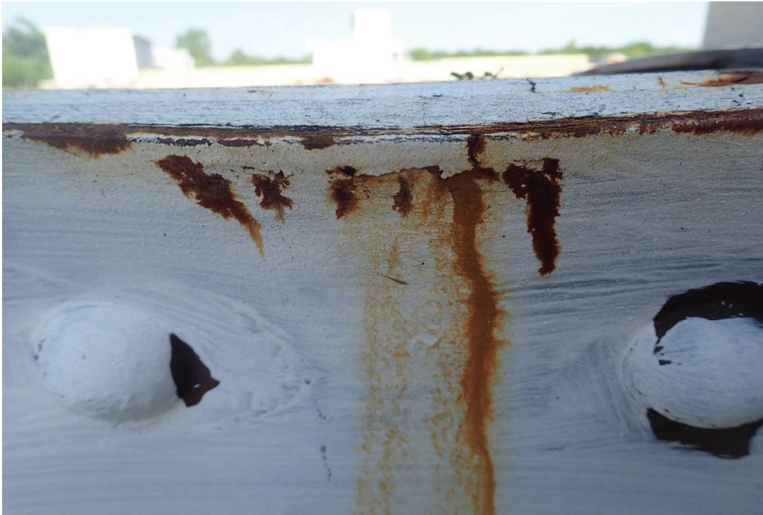
Photo 11: Small crack in web plate of Channel B at Cross Section 1
