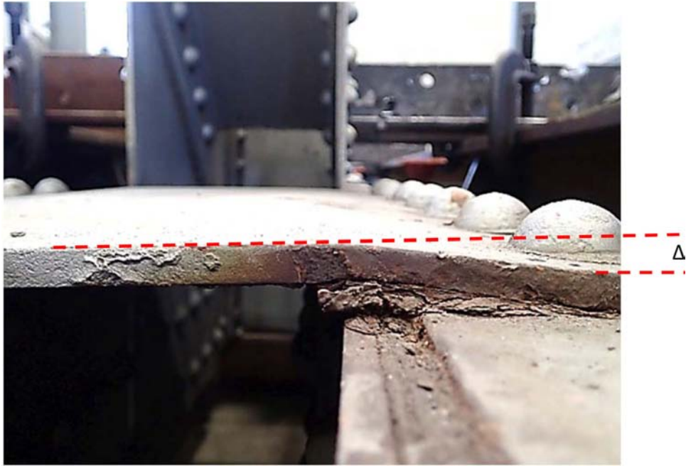
Figure 5.6 Specimen 1 end stay plate prior to testing showing pack rust-induced bending.
