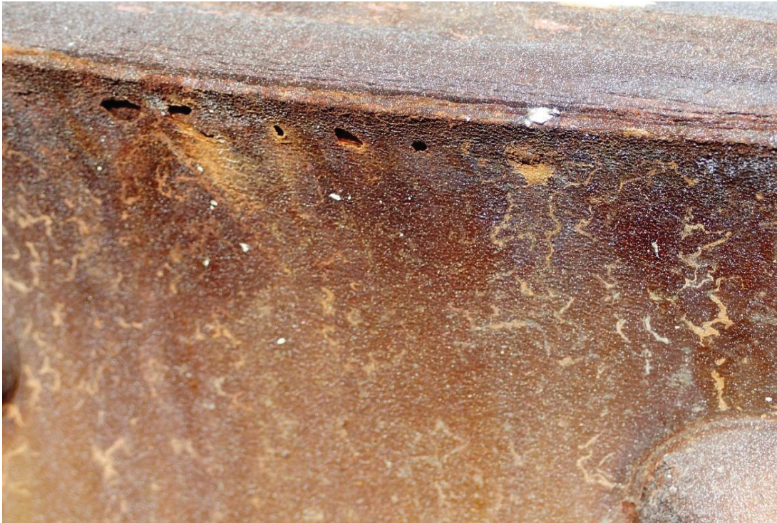
Photo 18: Small holes in web plate of Channel B near Cross Section 2
