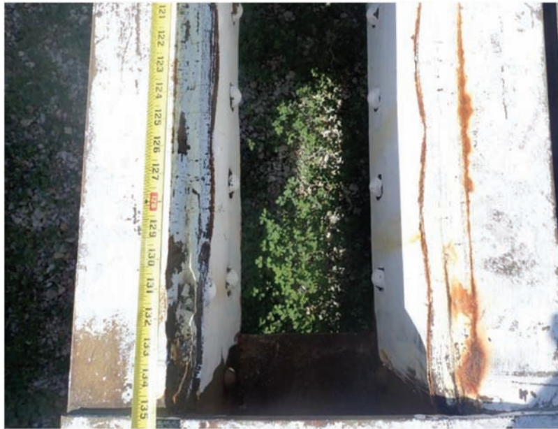
Figure 7.5 Region identified as the critical section by three of the inspectors.
