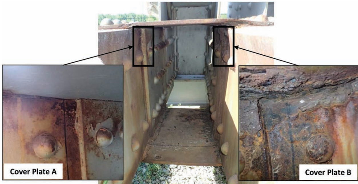
Figure 7.9 Cover plate condition at Cross Section 2.
