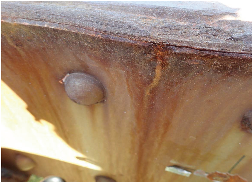
Photo 6: Crack in web plate near top (similar in a few locations)
