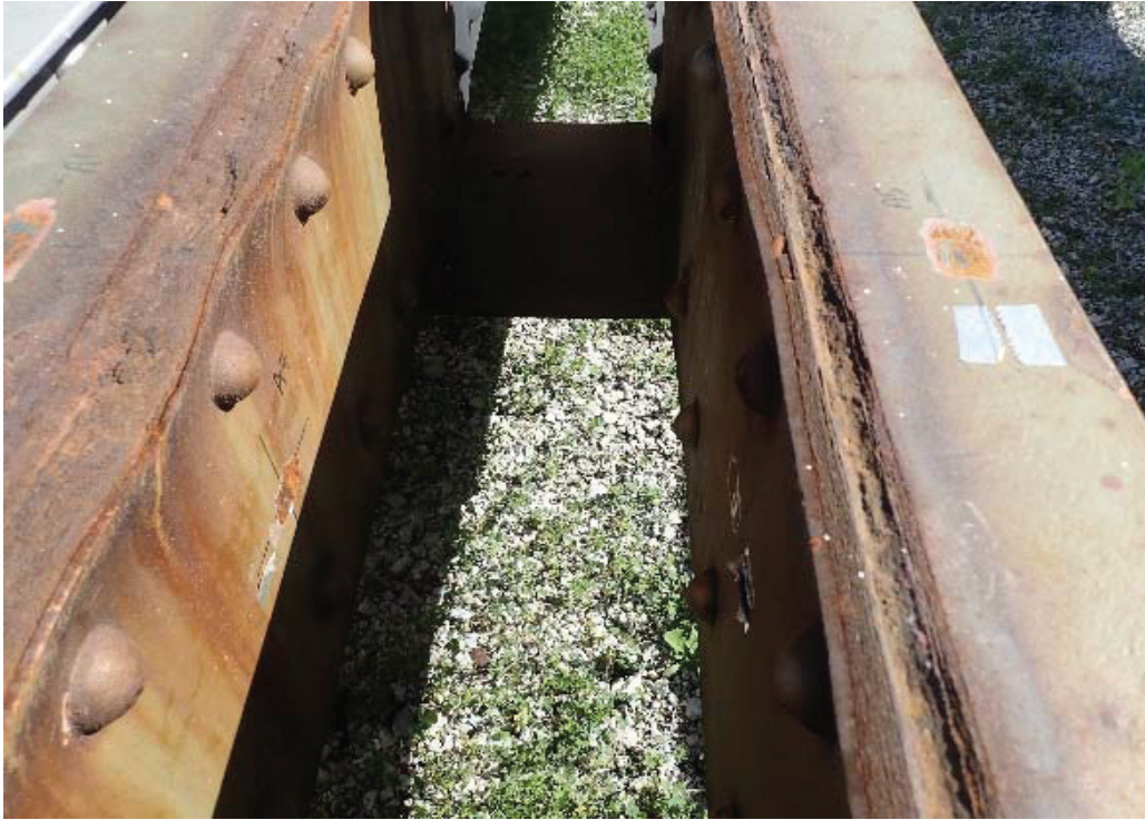
Photo 3: General condition of web plate and channels (looking from L2 to L4)
