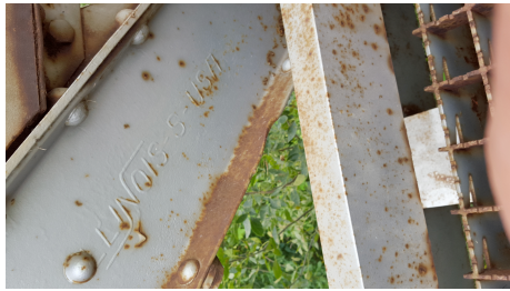
Fig. 26. Corrosion on truss elements
