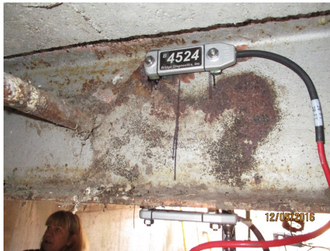
Fig. 48. Transducer attached to the top part of girder web at the same location as the bottom transducer
