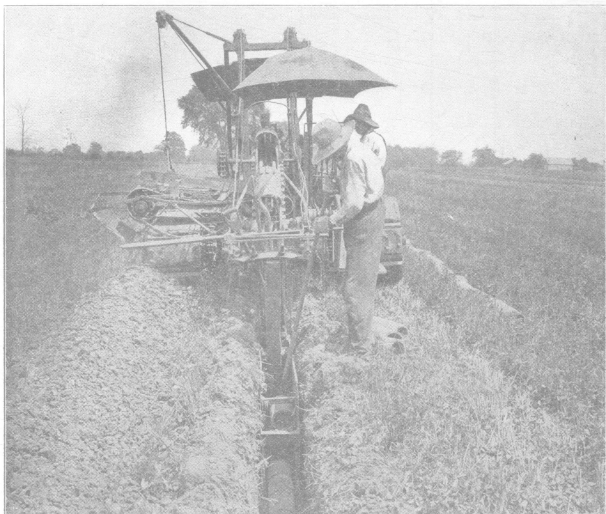
Fig. 5.—String the tile 6 feet to the right of the ditch line. Use a shield on the machine to keep the ditch bottom free from crumbs. These factors plus a tile hook make it possible for one man to keep up with a machine digging 150 rods per day.
