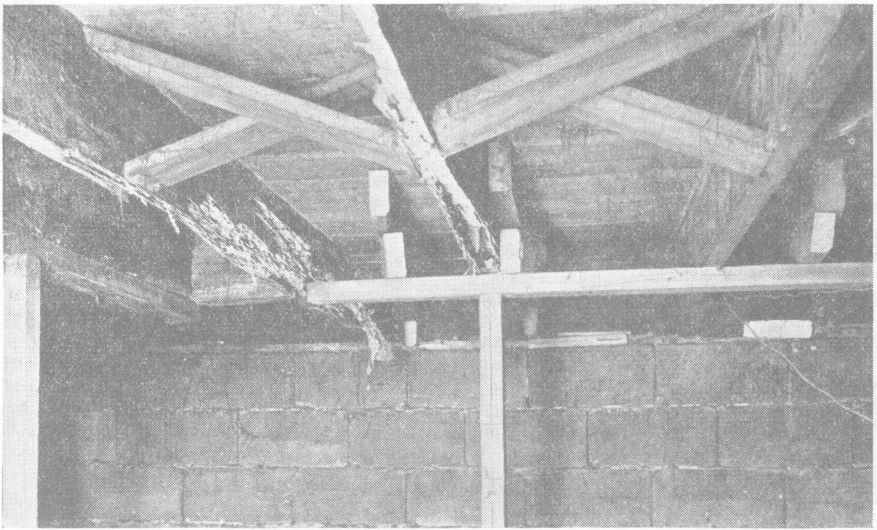
FIG. 1.—Typical termite damage to supporting timbers.
