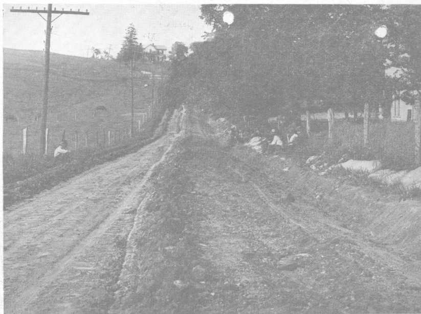
Fig. 9.—Loose earth of second and third rounds has been moved toward the center of road
