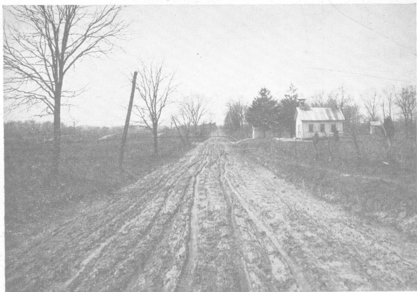
Fig. 17.—Graded road upon which maintenance has been neglected
