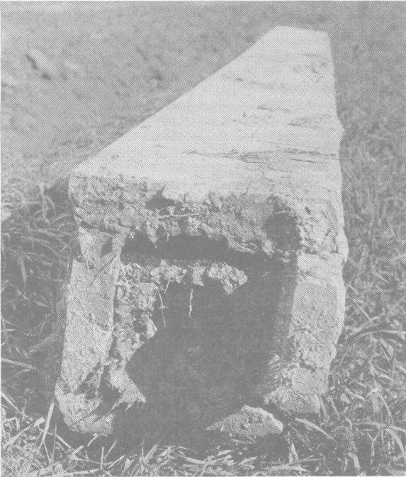
Fig. 1.—Culvert clogged with dirt, removed before grading
