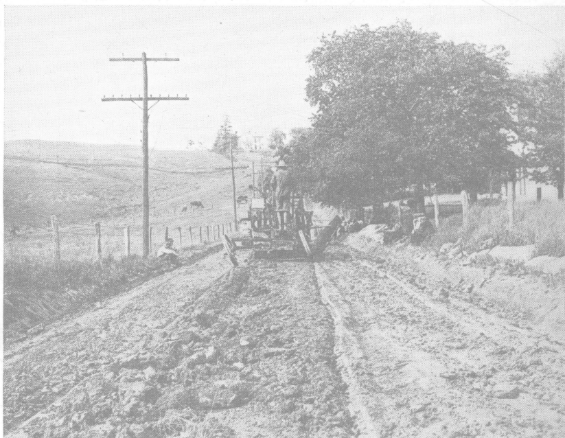
Fig. 12.—Transferring the loose earth of the former rounds to the center of the road
