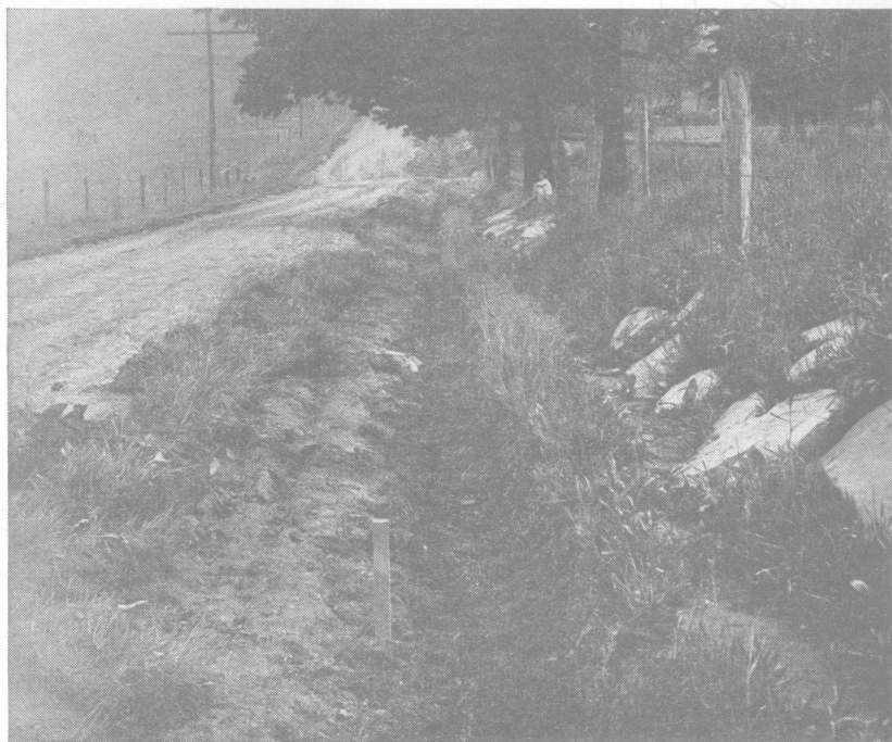
Fig. 5.—Sods removed from site of ditch to the shoulder line in the first round
