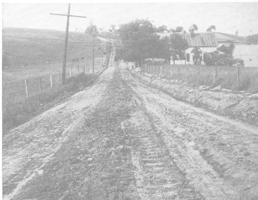
Fig. 13.—Grading operations completed. Several rounds of the road drag will give a smooth surface
