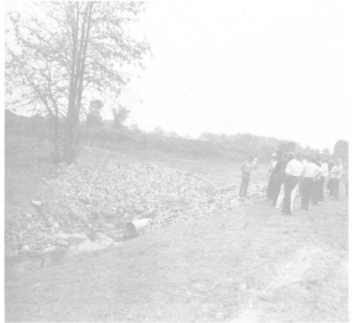
Upstream end of newly constructed drainage improvement showing outlet pipes and rock chute for erosion control.
