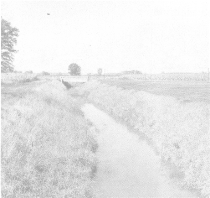
Well constructed drainage improvement project with good stand of vegetation (Auglaize County).
